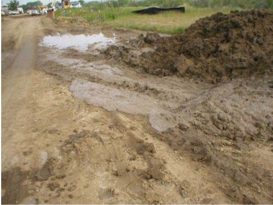
Figure 3 - New Vineyard Road Tributary tie-in work. Note the large mud pile to the right of the photo.
