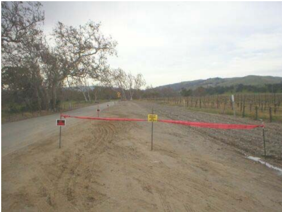
Figure 4 – Fencing and additional signs installed at the Red Tail Hawk's nest exclusion boundaries.
