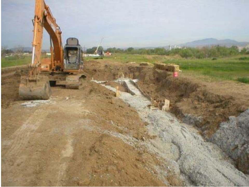
Figure 1 - New Vineyard Road Tributary tie-in work, the HDPE casings and conduit have been poured in concrete.
