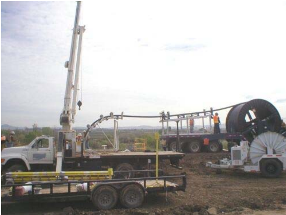
Figure 2 - Transmission line pull from Vault 12 to Vault 11 through HDPE casings installed in the New Vineyard Road Tributary Bore.
