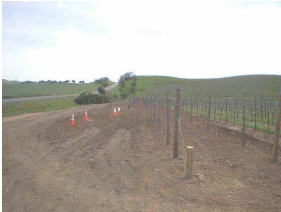
Figure 1 – Restoration work along the right-of-way. The area has been graded and new vine rows have been installed up to the underground installation.
