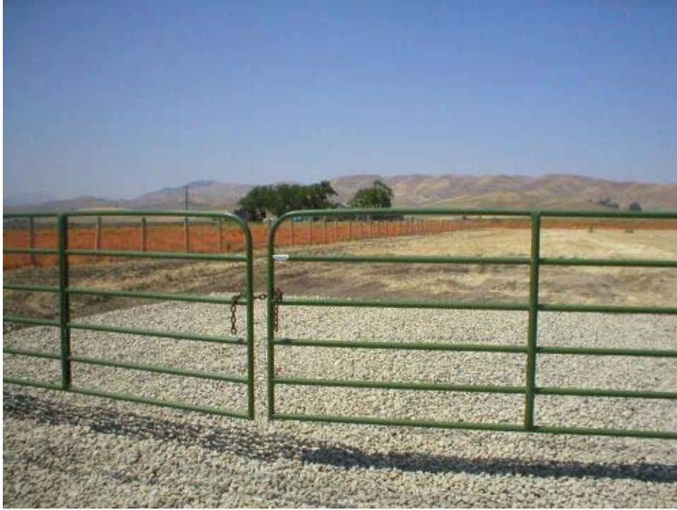
Figure 2 – May School Road lay down yard, Phase Two. The area has been mowed and gravel installed in the entrance area. The perimeter of the yard was disked and fencing was installed.
