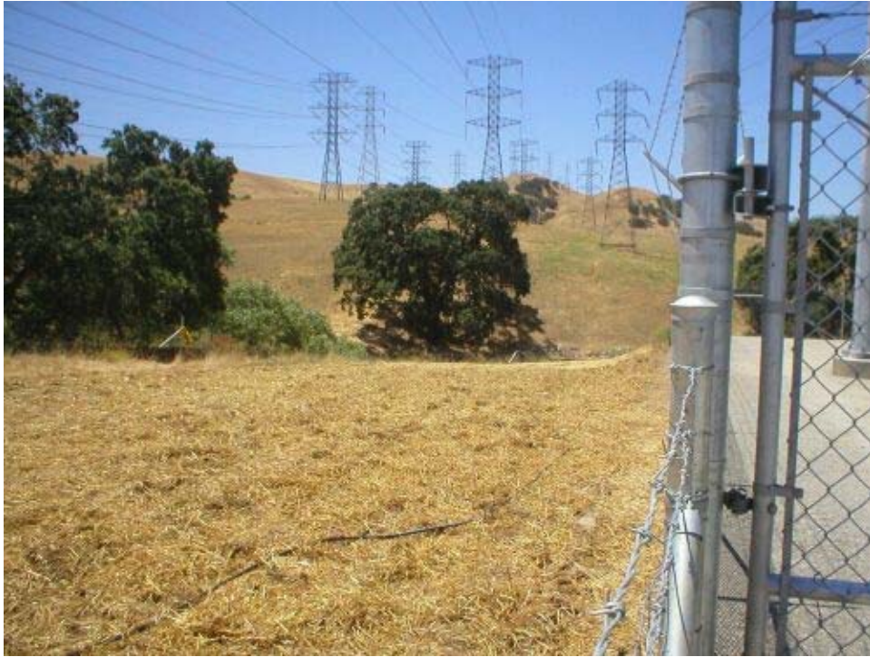
Figure 1 – At the Transition Station, the contractor has ripped the ground surface to a depth of six inches. The area was seeded and a mulch cover was applied. Crews continue to water the area. Phase One.
