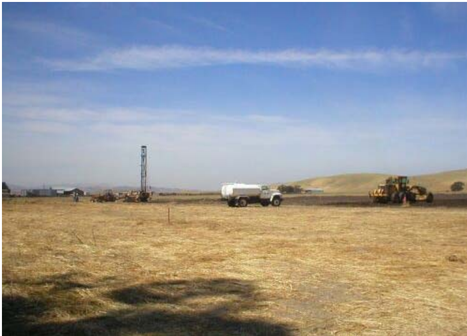
Figure 2 – Grading at the Cayetano Substation site. The structure to the left of the photo is a water well drill. Phase Two.
