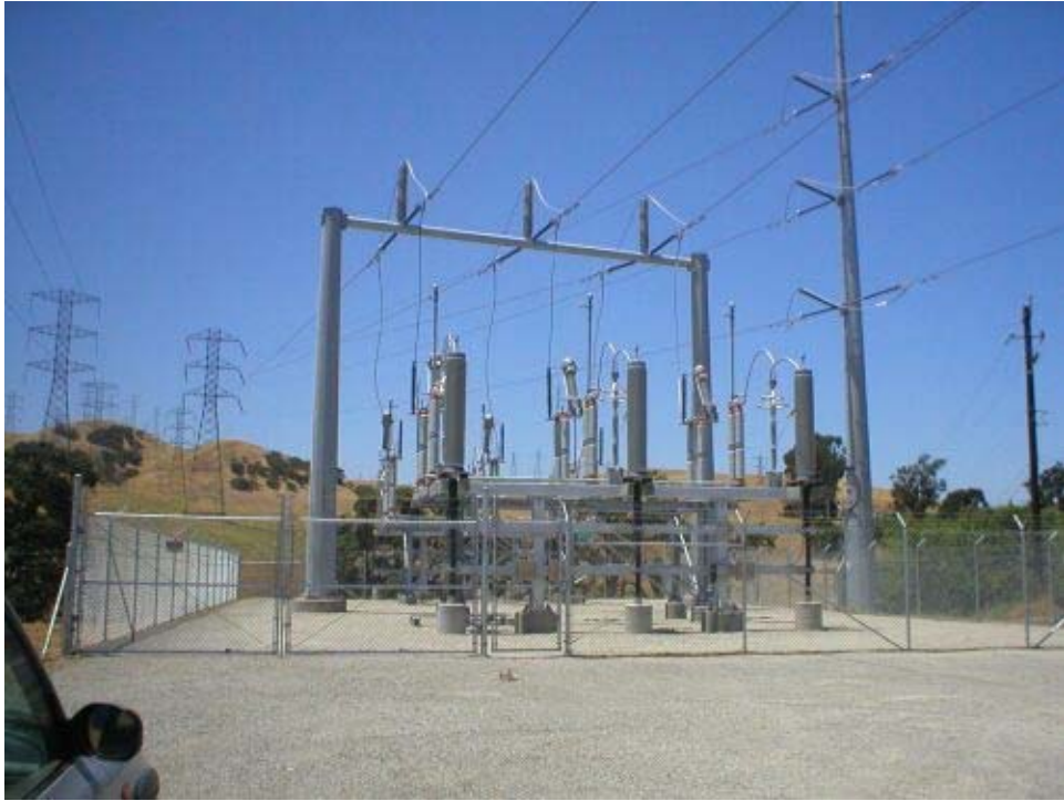
Figure 1 – Transition Station, Phase One.
