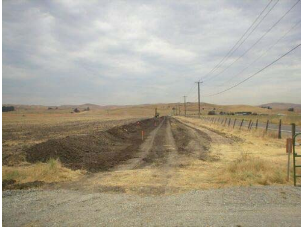
Figure 1 – Trench line preparation between Dagnino Road and the PSD Yard, Phase Two. Crews have begun scraping the topsoil layer to the side of the trench.
