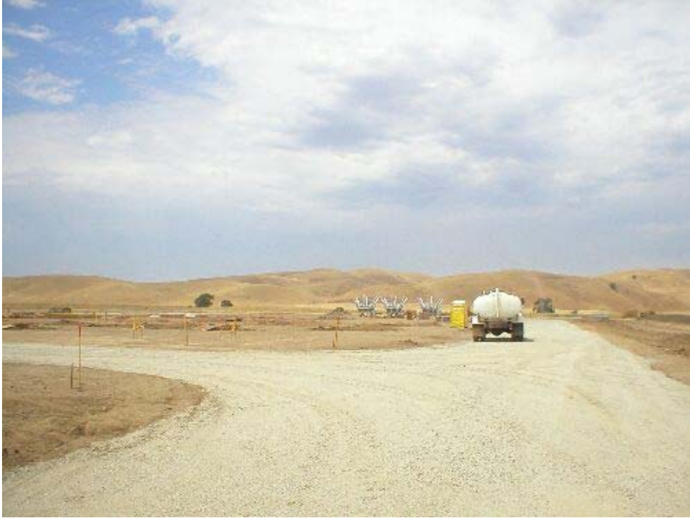
Figure 1 – Cayetano Substation, Phase Two.
