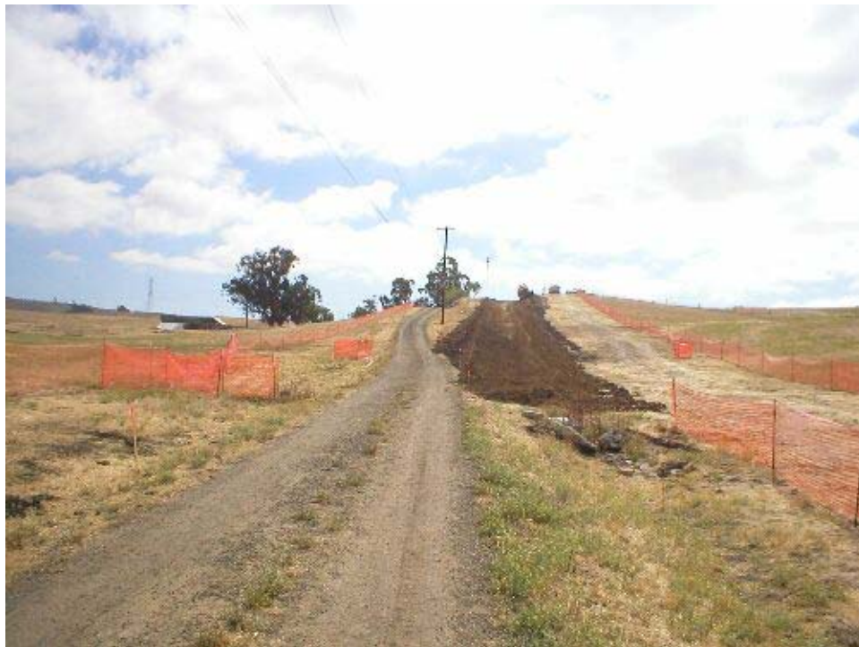
Figure 2 – Access road construction between Dagnino Road and the Transition Station, Phase Two. Note that the road construction did not cross the drainage in the foreground.
