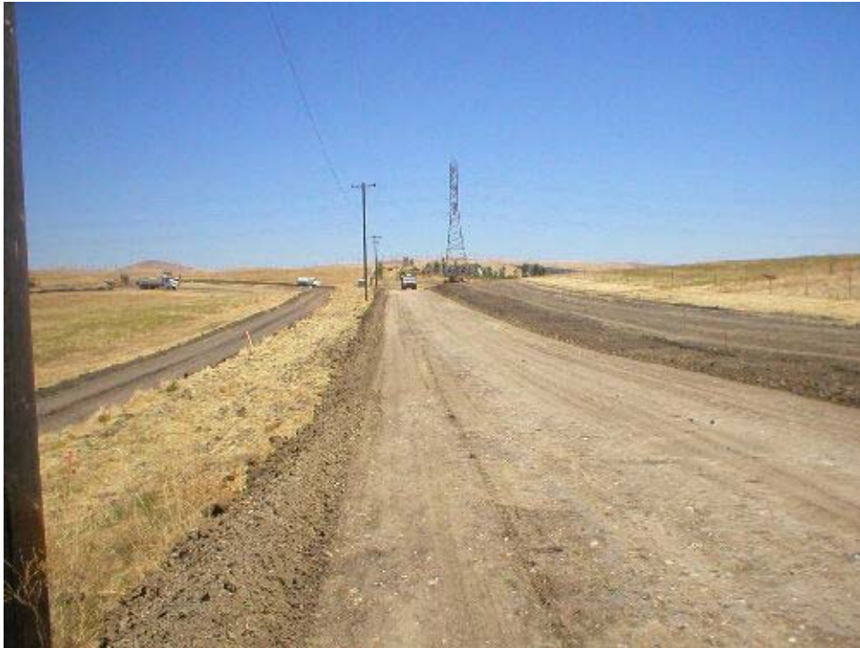
Figure 3 – Access road construction between Dagnino Road and the Transition Station, Phase Two. Note the center strip is the new road, directly to the right of the road is a parallel graded firebreak.
