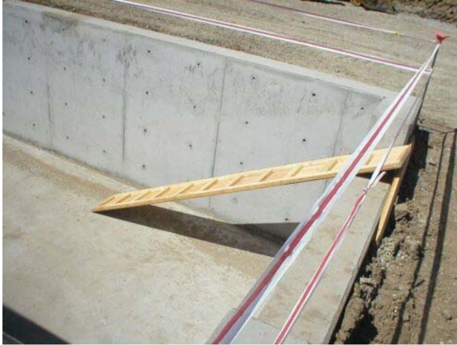
Figure 1 – Ramp installed for San Joaquin Kit Fox and other wildlife protection within the SPCC pond built at the Cayetano Substation, Phase Two.
