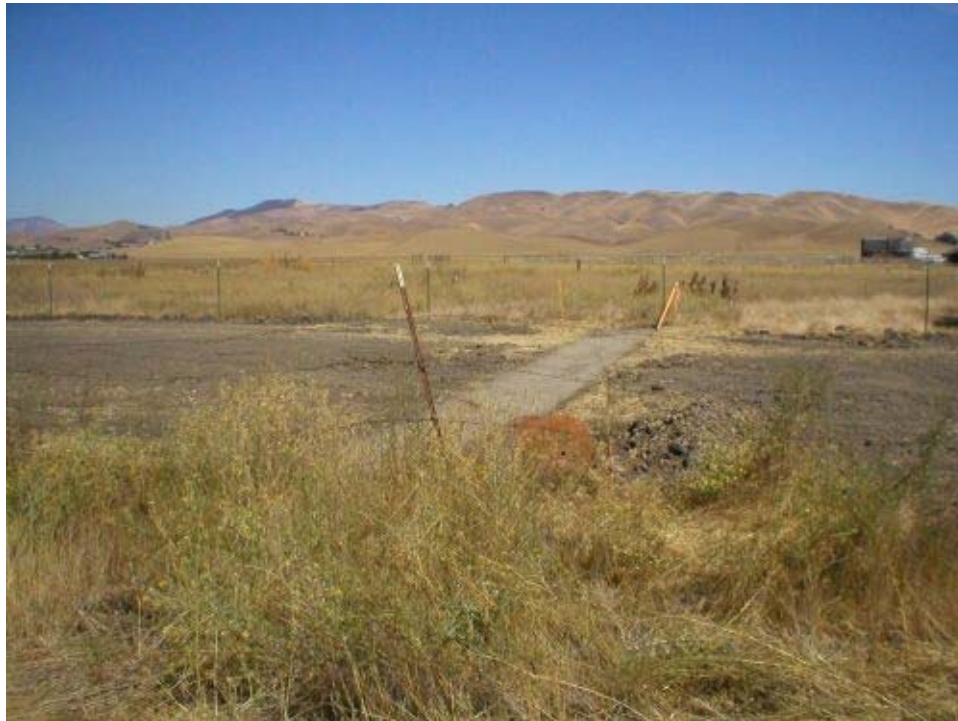
Figure 2 – Trenching and conduit installation under the UAD along May School Road is complete. The contractor has backfilled soil up to the cultural resource , Phase Two.
