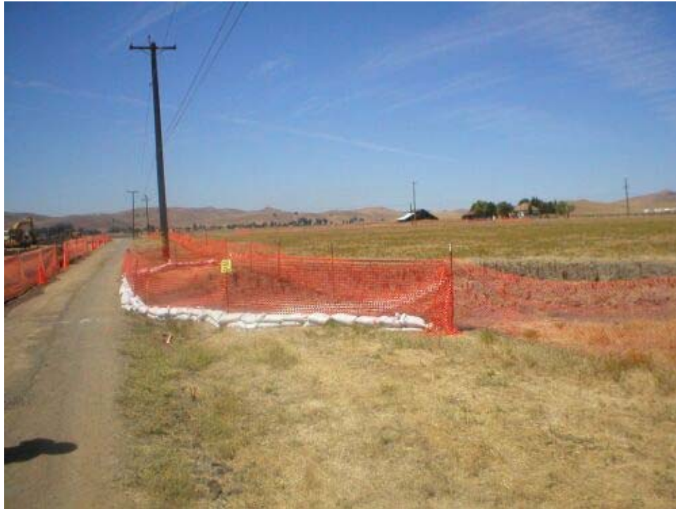
Figure 3 – Reduced buffer zone for wetland habitat along the North side of the access road between Dagnino Road and the Transition Station, Phase Two. The PG&E trench line is on the opposite side of the access road from the resource.
