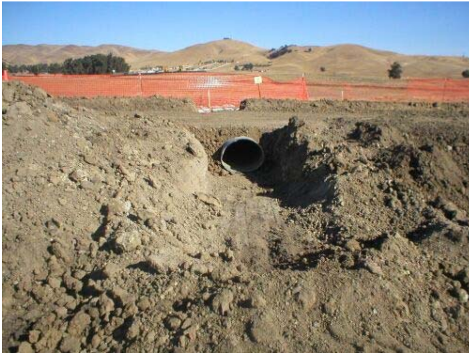
Figure 2 – New culvert installed under the access road being upgraded east of Dagnino Road, Phase Two.
