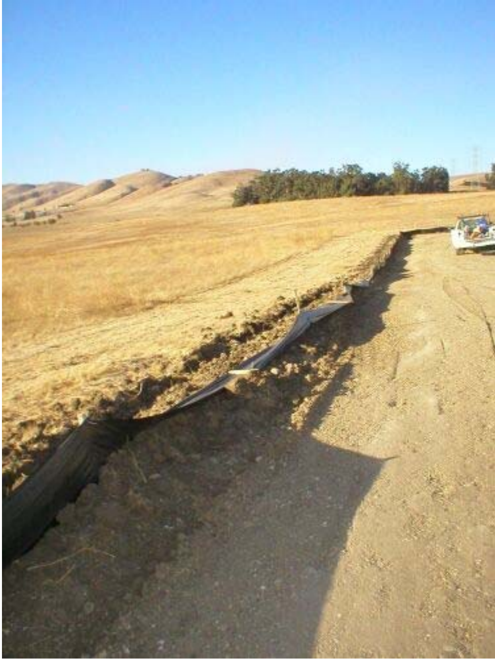
Figure 1 – Sediment fence in need of repair along the west side of the Transition Station., Phase Two.
