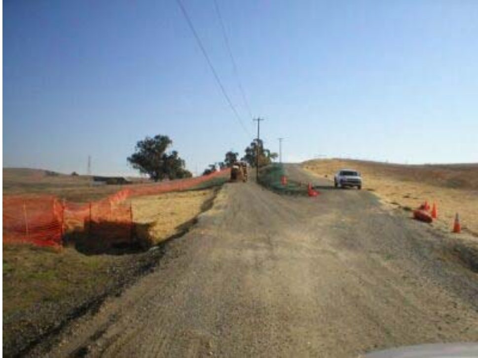
Figure 3 – Hydro seeding and mulch cover along the access road to the Transition Station, Phase Two.
