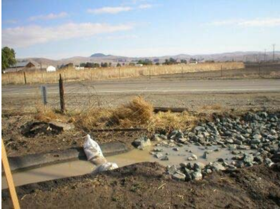
Figure 1 – Muddy water runoff from the Cayetano Substation, Phase Two.
