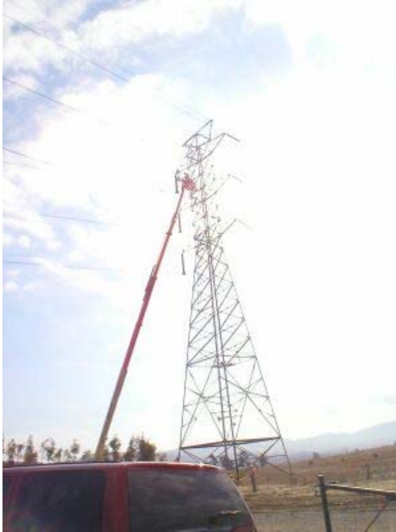
Figure 5 – Grounded Contra Costa-Newark Circuit line transfer to the Transition Station, Phase Two.
