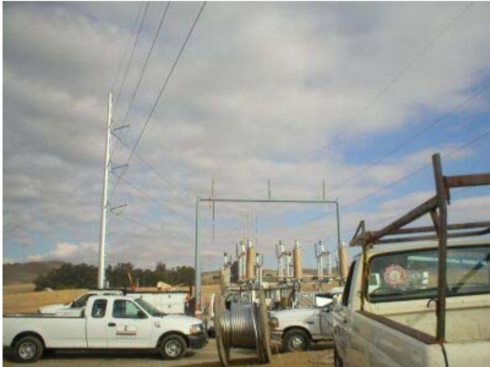
Figure 4 –Transition Station H-frame structure, Phase Two.
