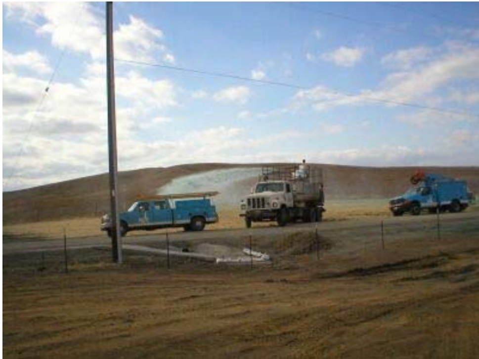
Figure 2 – Hydro seeding along the access road to the Transition Station, Phase Two.
