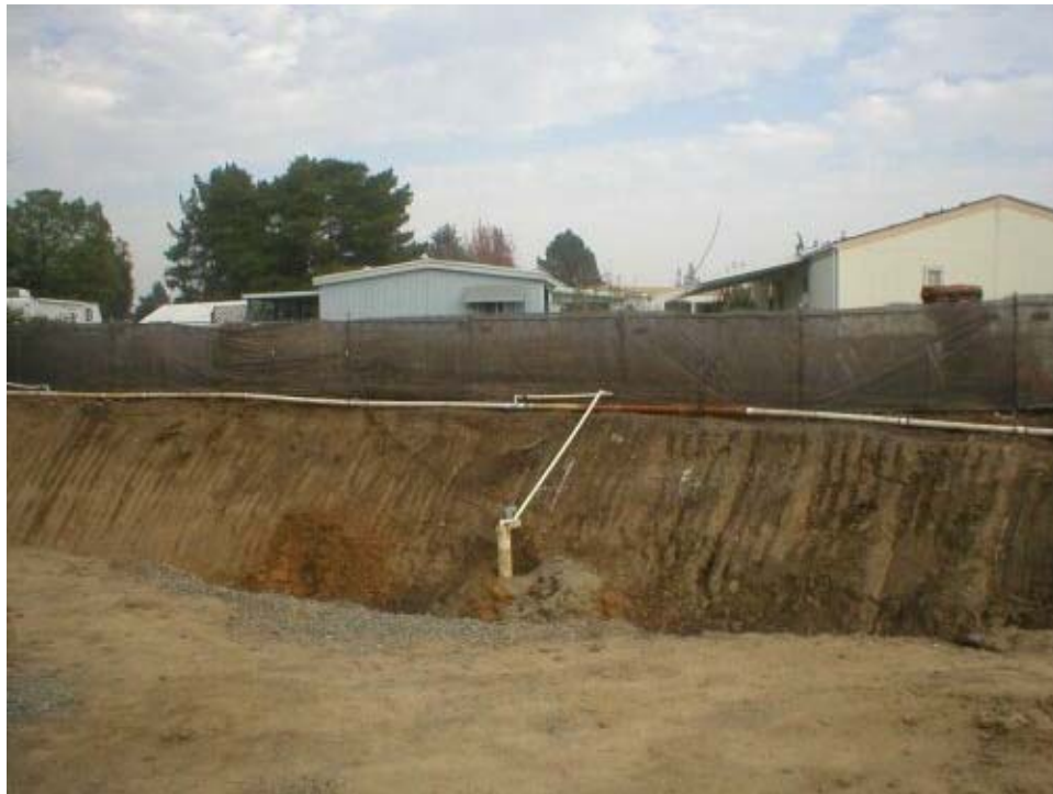
Figure 1 Pilot wells and de-watering piping installations at the Arroyo del Valle south bore pit.
