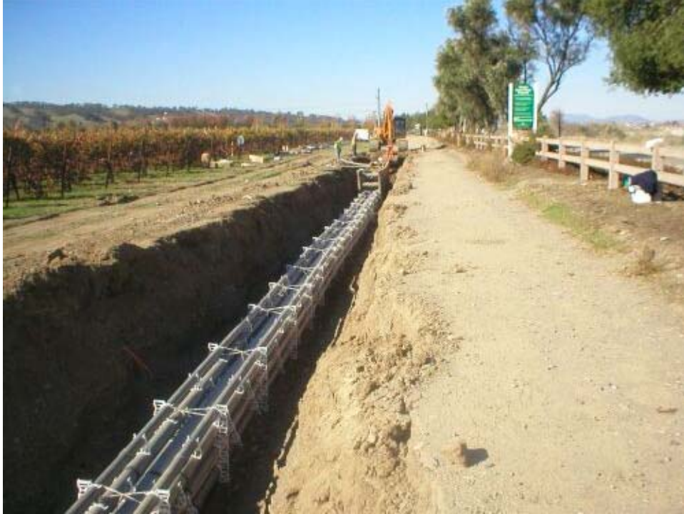
Figure 2 Trenching and conduit installation along “Old” Vineyard Avenue west of Isabel Avenue.
