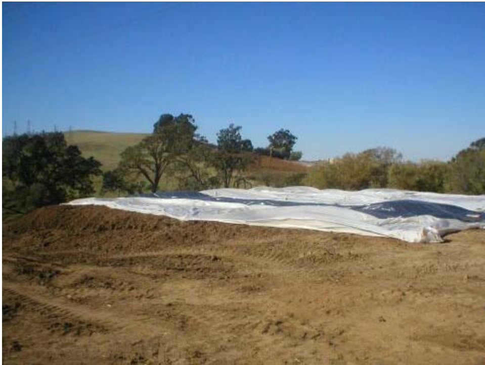
Figure 3 Continued work and grading at the Transition Station. Prior to the Thanksgiving break, visquene was placed over the landing on site.
