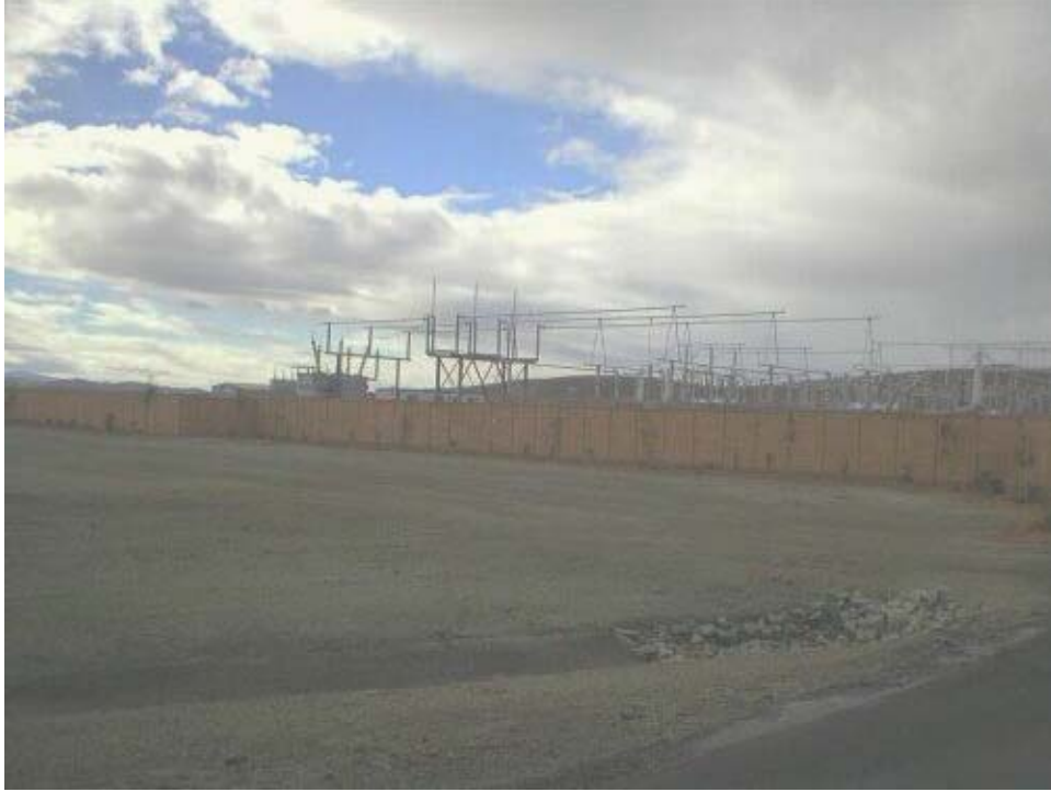
Figure 1 – The area surrounding the Cayetano Substation has been hydro-seeded, Phase Two
