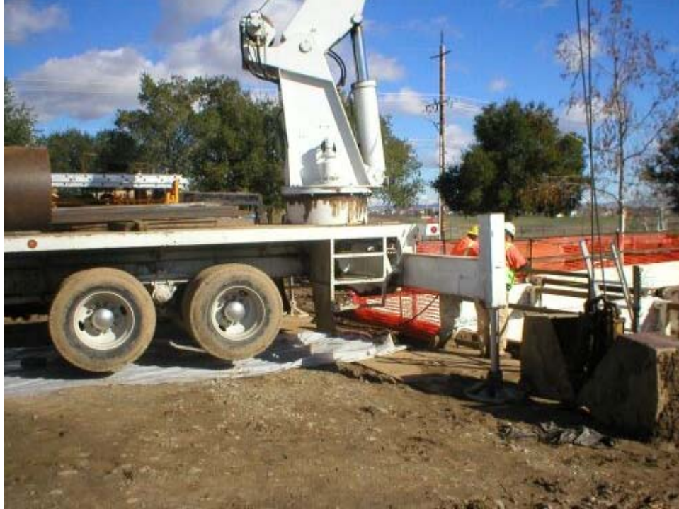
Figure 2 Ruby Hills west bore pit. The crane pictured had been leaking hydraulic fluid; the material was cleaned up and plastic was placed underneath the equipment.
