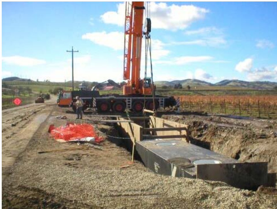
Figure 3 Vault 4A and 4B construction adjacent to the Zone 7 Access Road. Note the large amount of dirt and mud tracked into the road.
