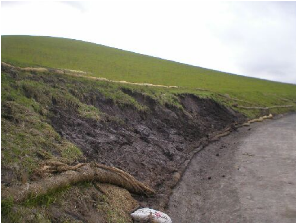
Figure 1 – Continued slumping along Road 6, March 24, 2006.
