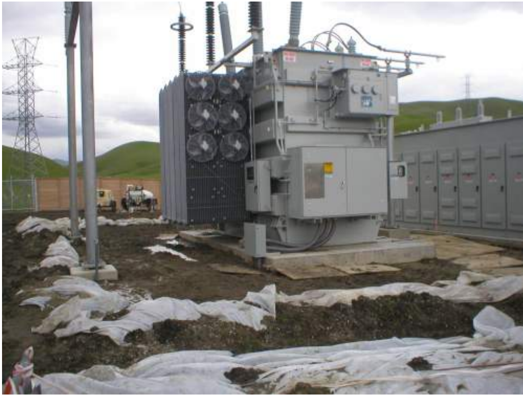
Figure 3 – Transformer surrounded by an earthen berm at the North Dublin Substation, March 30, 2006.
