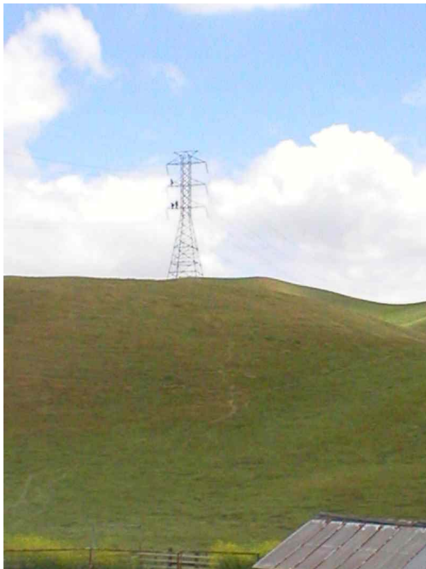
Figure 1 – PG&E crews installing bird guards at Tower #2. Please note the foot-path utilized to access the location, May 22, 2006.
