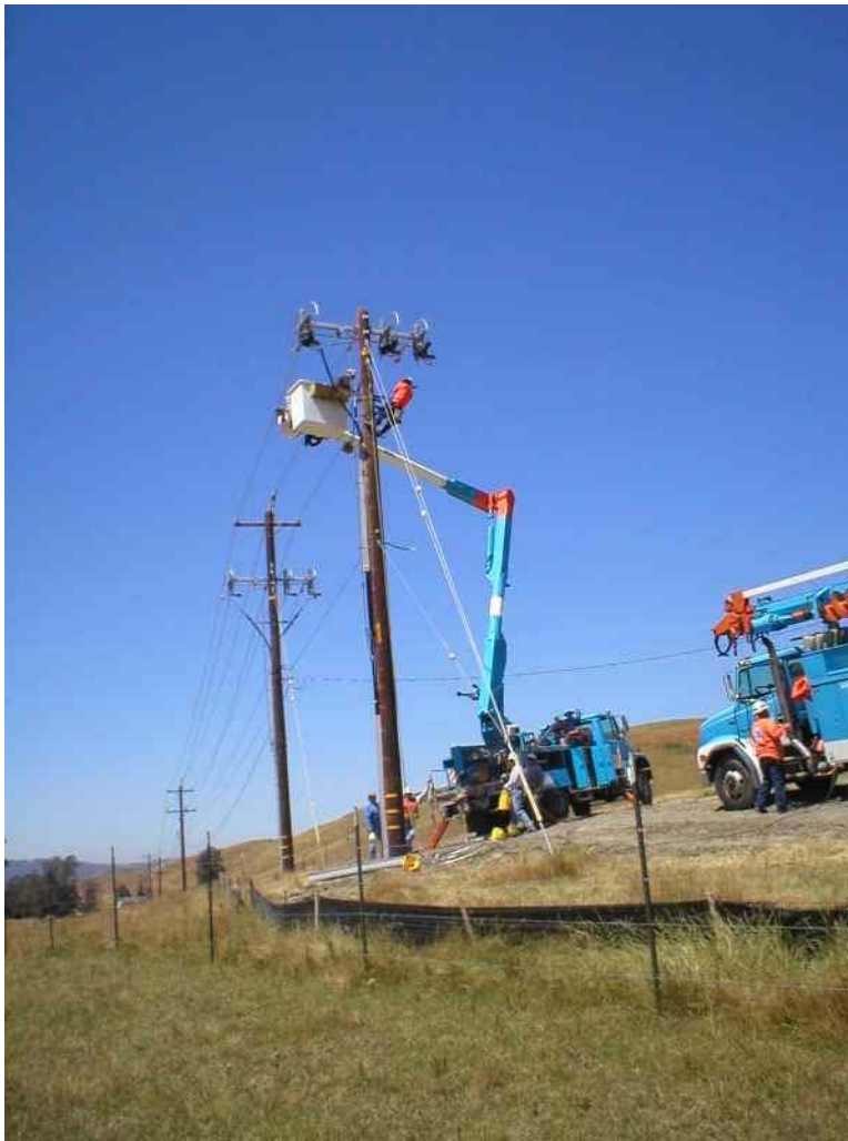
Figure 3 – PG&E crew stringing a distribution line which connects to the North Dublin Substation, June 6, 2006
