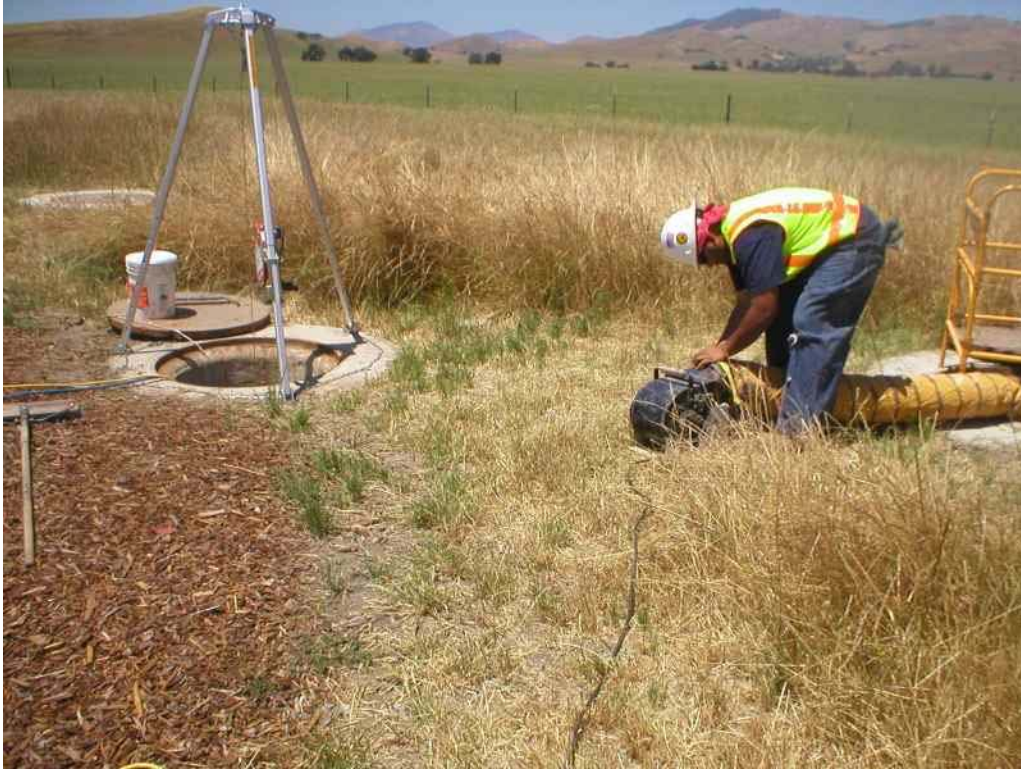
Figure 1 – Jenson PreCast working at Vault 1. Within the underground vault crews continue racking in preparation for the transmission line stringing and splicing, June 6, 2006.
