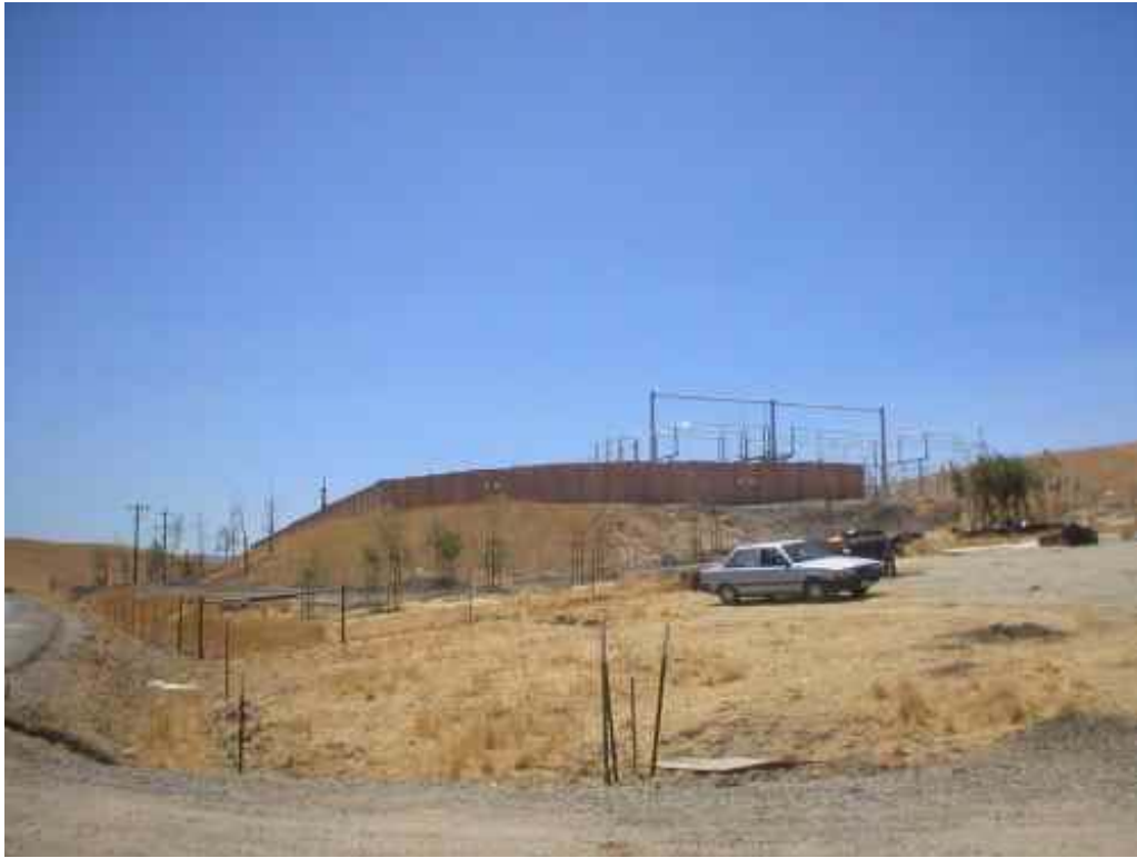
Figure 3 – Landscape plantings around the North Dublin Substation, July 25, 2006.
