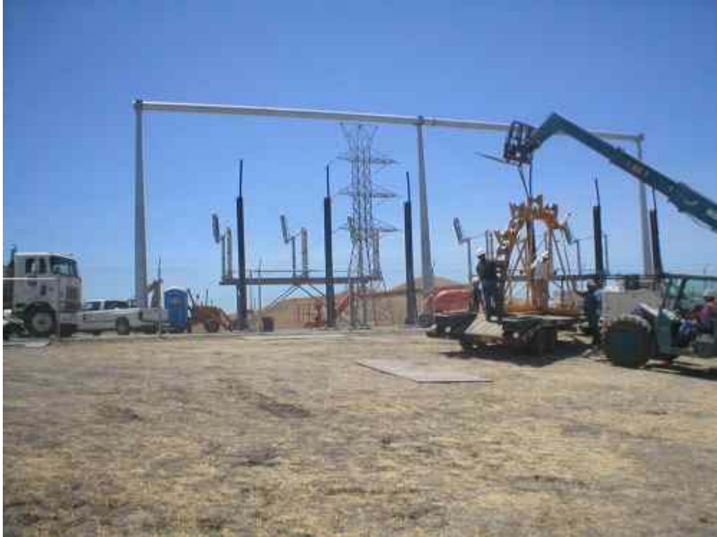
Figure 1 – Cable pulling operations at Vault 8 next to the Transition Station were completed and crews are shown de-mobilizing from the site. July 25, 2006.
