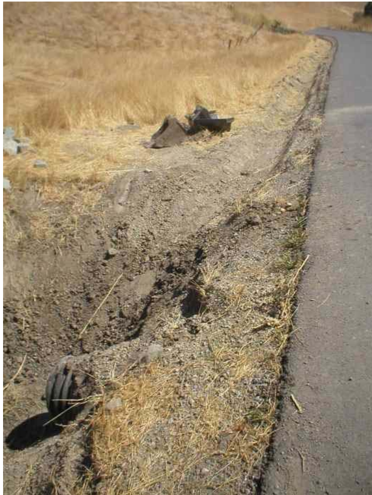
Figure 4 - NVC cleaned out culverts and v-ditch area along Moller Road during restoration activities, August 10, 2006.
