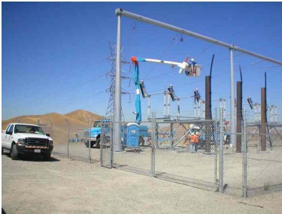
Figure 2 – Transition Station, August 10, 2006.
