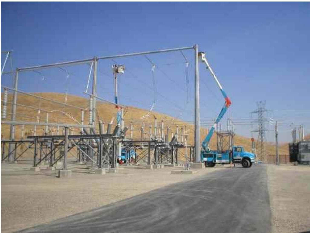
Figure 5 – PG&E crew working on the frame structure at the North Dublin Substation, September 7, 2006.
