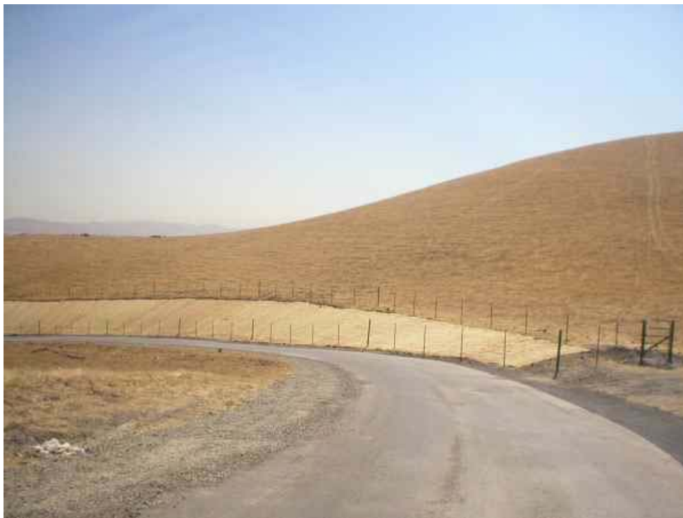
Figure 2 – NVC crews fenced around the side slope restoration area along Road 6, September 13, 2006.
