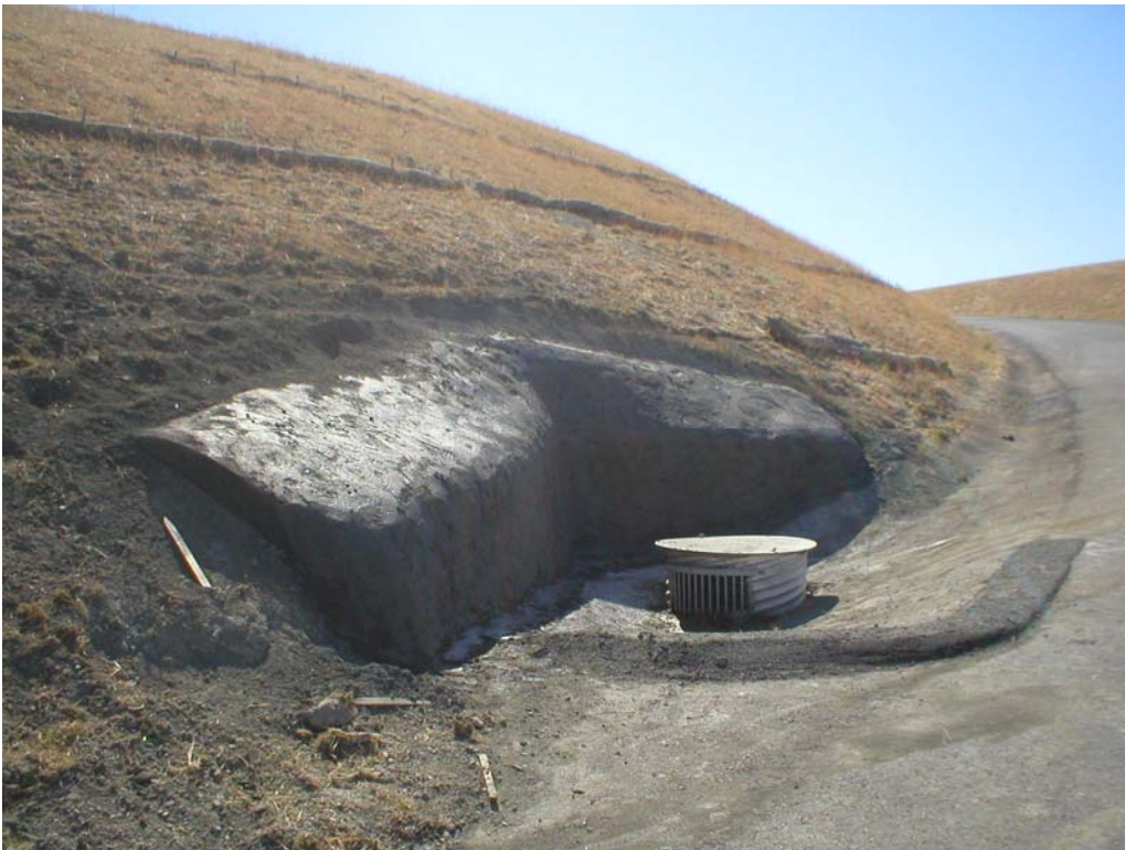
Figure 2 – NVC crews placed asphalt around the rebar installed at a culvert area along Road 6, September 18, 2006.
