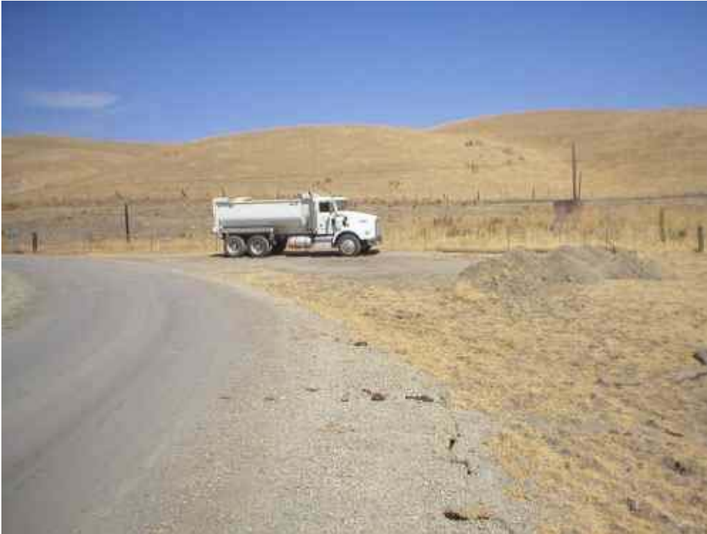
Figure 1 – Turnaround area being created by NVC as requested by the landowner, September 18, 2006.
