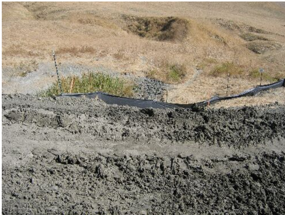
Figure 3 – Sediment fencing in need of repairs and removal of spoils along Moller Road, August 31, 2005.
