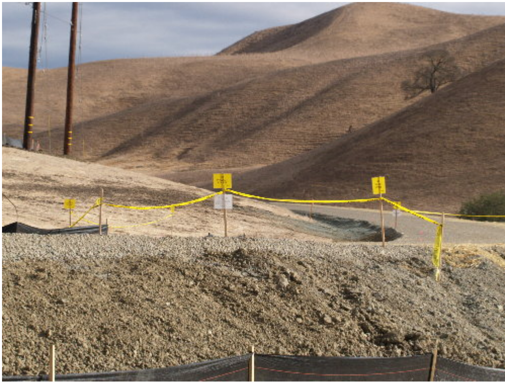
Figure 6 – Exclusion tape and signs were placed on a section of Moller Ranch Road within 160 feet of the burrowing owl burrow discovered on October 27 th .
