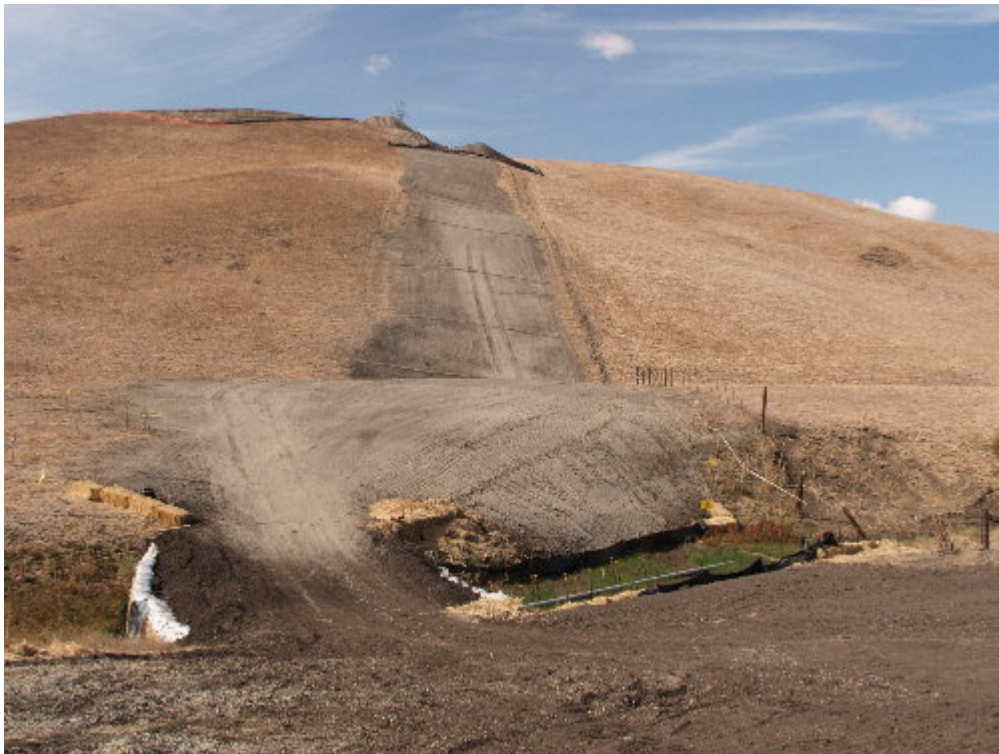
Figure 4 – Long slope over Cayetano Creek lacks adequate BMPs to address erosion prevention and sediment control.
