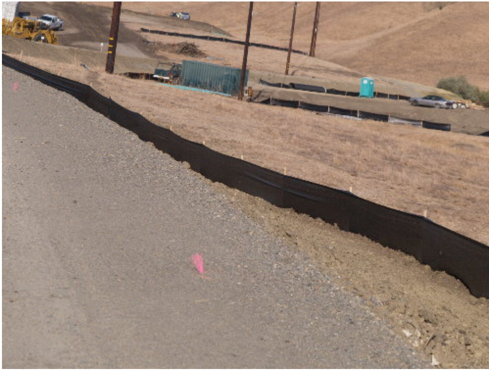
Figure 5 – The silt fencing in several locations was installed either too tightly or at an angle allowing water and sediment to flow along the silt fencing towards resources.
