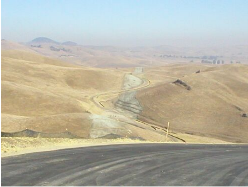
Figure 2 – Road 7 and trench line, November 18. Note the lack of erosion controls over the trench line.
