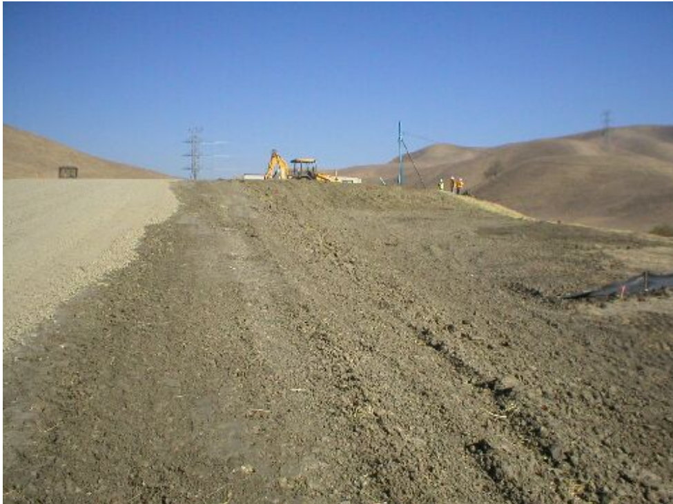
Figure 4 – Work to extend the Substation pad, November 22, 2005. Note the buried sediment fence to the right.
