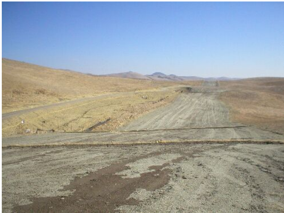
Figure 2 – Road 7 and trench line, November 22, 2005. Note the sparse erosion controls over the trench line.
