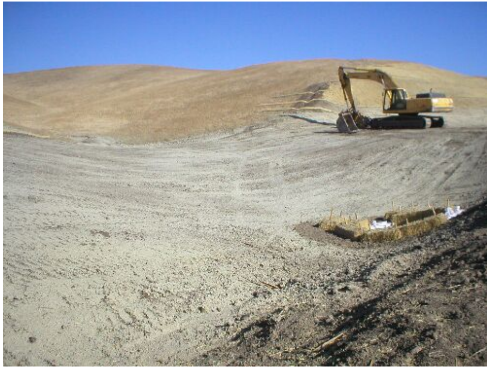
Figure 3 – Road 7, trench line and culvert area, November 22, 2005. Note the sparse erosion controls.
