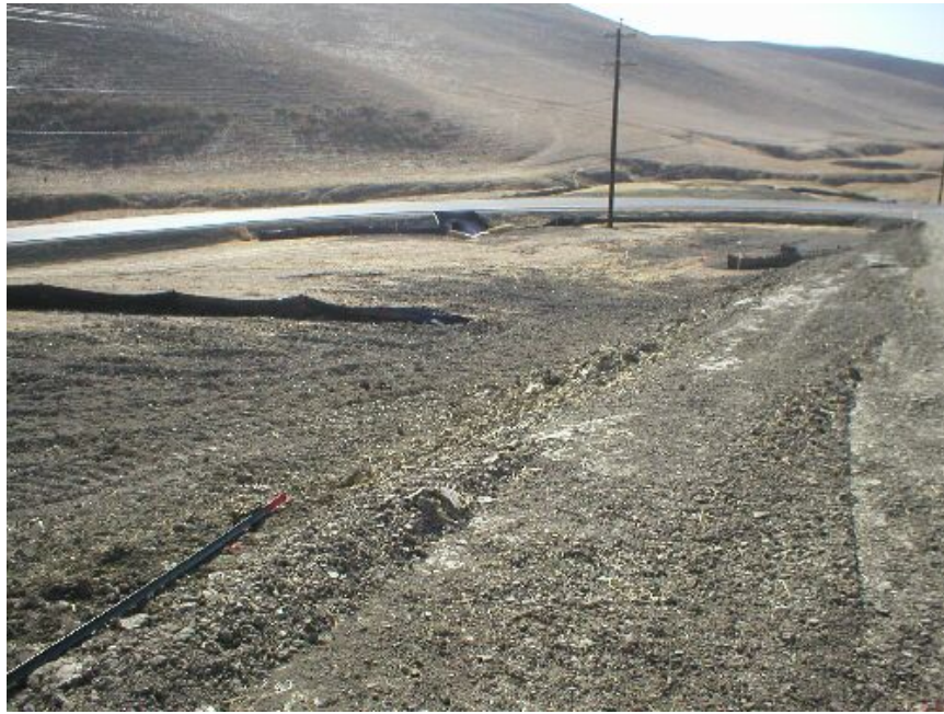
Figure 5 – Work to extend the Substation pad, November 22, 2005. Note the buried sediment fence to the left and the culvert.
