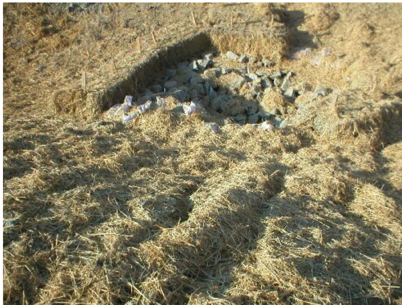
Figure 2 – Area of erosion near a culvert along Road 7, December 8, 2005. Hay was broadcast and the area hydro-seeded during the subject week.
