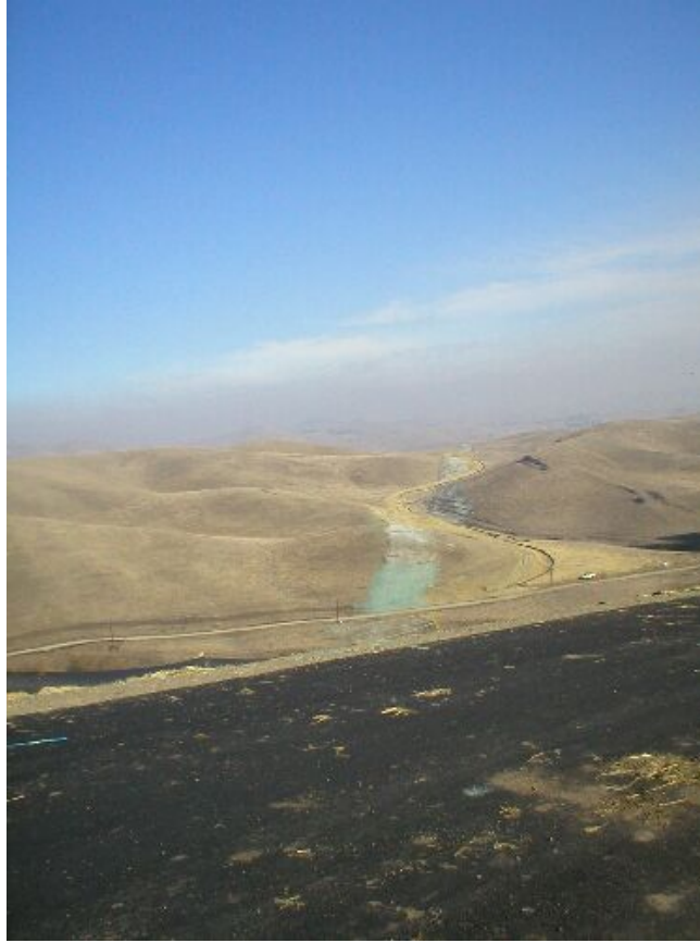
Figure 1 – Trench line extending from the Transition Station and Road 7, December 8. Note the new, green hydro-seed.
