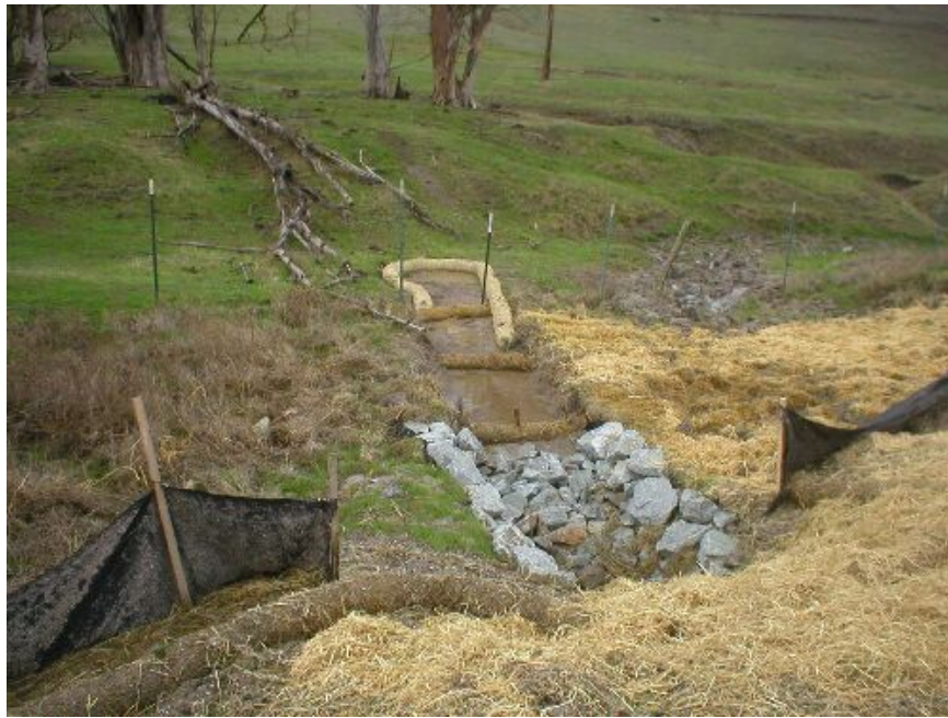
Figure 5 – Sediment cleaned and contained past a culvert along Moller Road upstream of Tassajara Creek , December 22, 2005.
