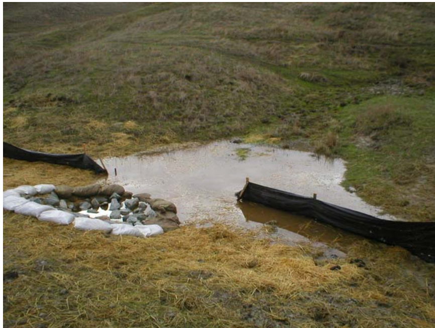
Figure 3 – Flooded culvert inlet located along the MSA Access Road, December 19, 2005.
