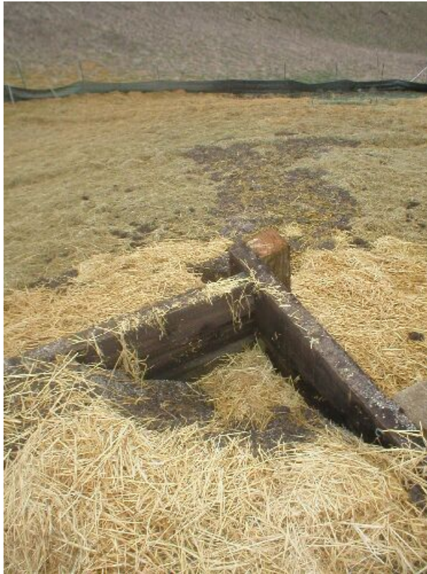
Figure 2 – Erosion at the Transition Station bulkhead, December 20, 2005.
