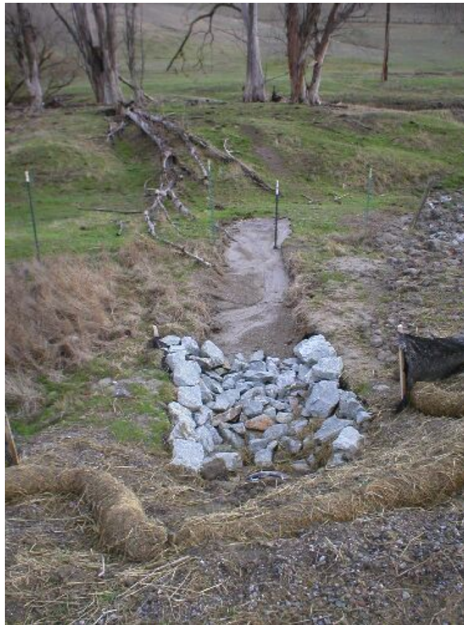
Figure 4 – Sediment past a culvert along Moller Road upstream of Tassajara Creek, December 19, 2005.
