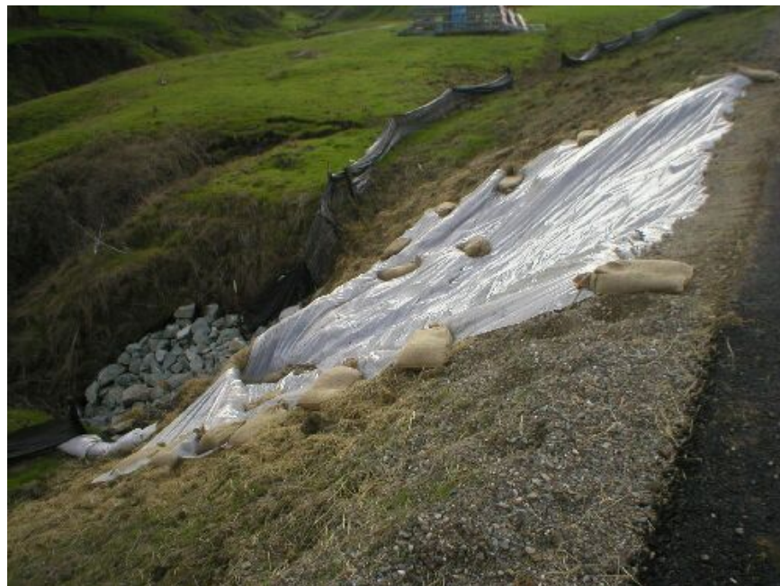
Figure 4 – Plastic placed over a small landslide at a culvert outlet along Moller Road, January 13, 2006.
