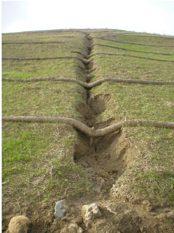
Figure 3 – Erosion along the earthen v-ditch along Moller Road, January 4, 2006.
