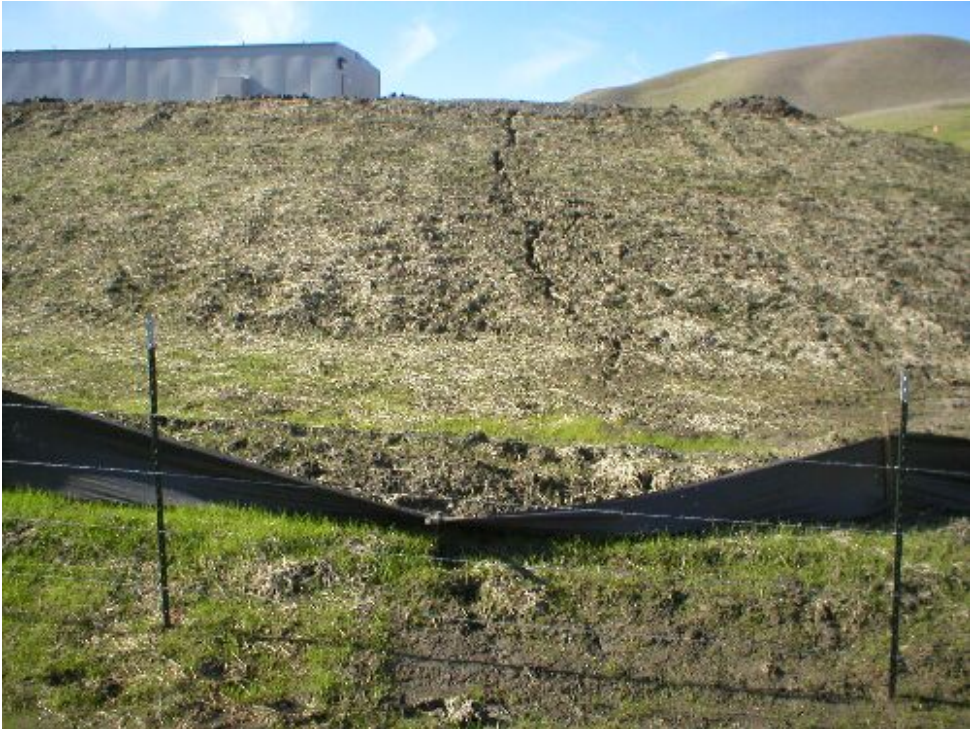
Figure 1 – Erosion extending down the side of the North Dublin Substation pad, January 20, 2006.
