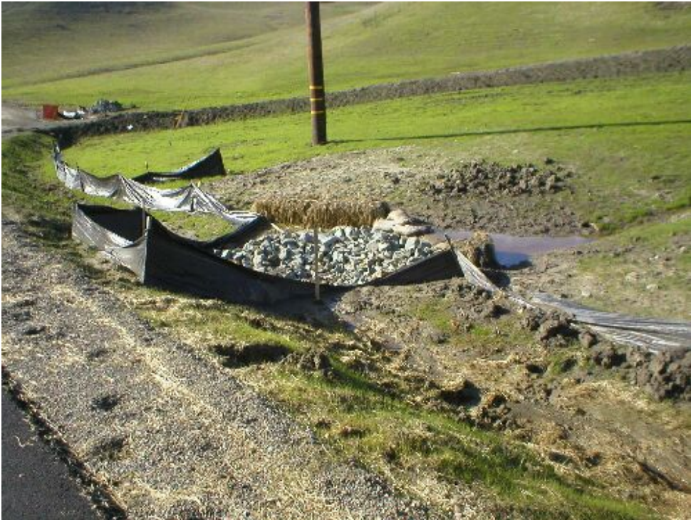
Figure 2 – Culver along Moller Road down slope of the substation in danger of being overrun by built-up sediment, January 20, 2006.
