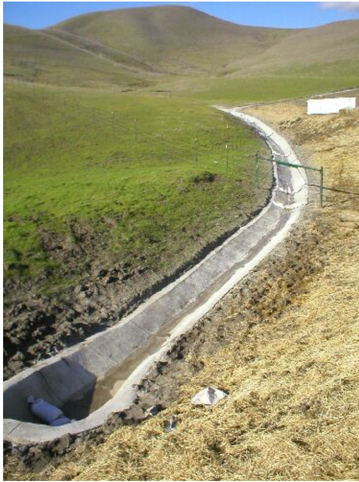
Figure 3 – Concrete lined v-ditch along the side of the North Dublin Substation, January 20, 2006.
