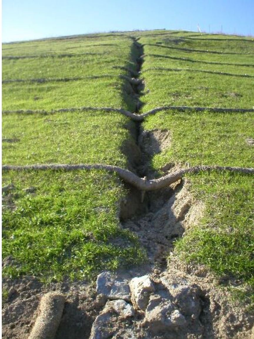
Figure 1 – Eroded v-ditch along Moller Road - February 9, 2006.
