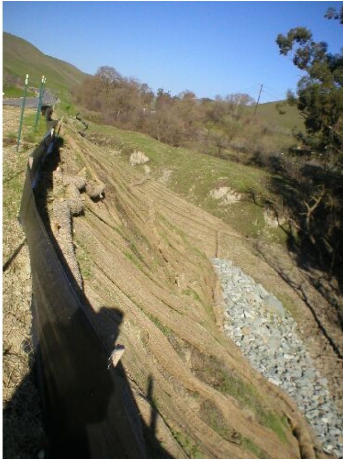
Figure 3 – Tassajara Creek bank stabilization area – February 9, 2006. Note the poor grass growth.
