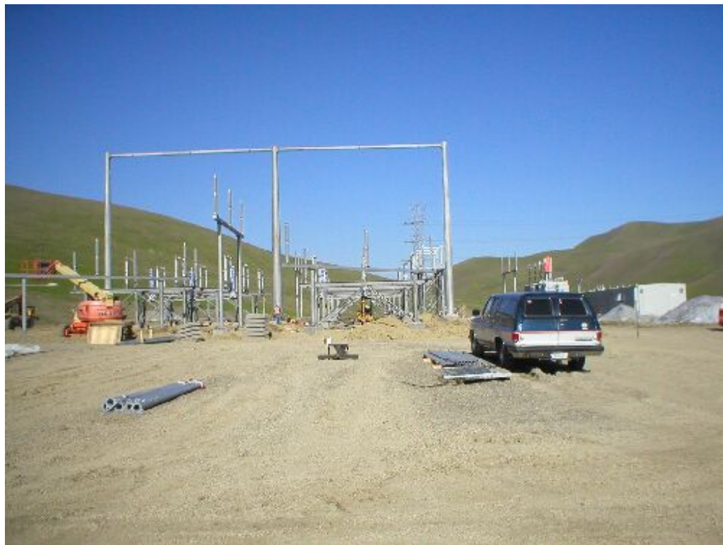
Figure 5 – North Dublin substation where trenching and grounding line installation is occurring - February 9, 2006.
