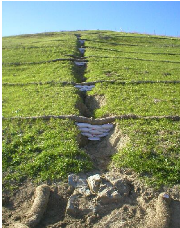
Figure 2 – Eroded v-ditch along Moller Road showing the newly installed sandbag check dams February 9, 2006.
