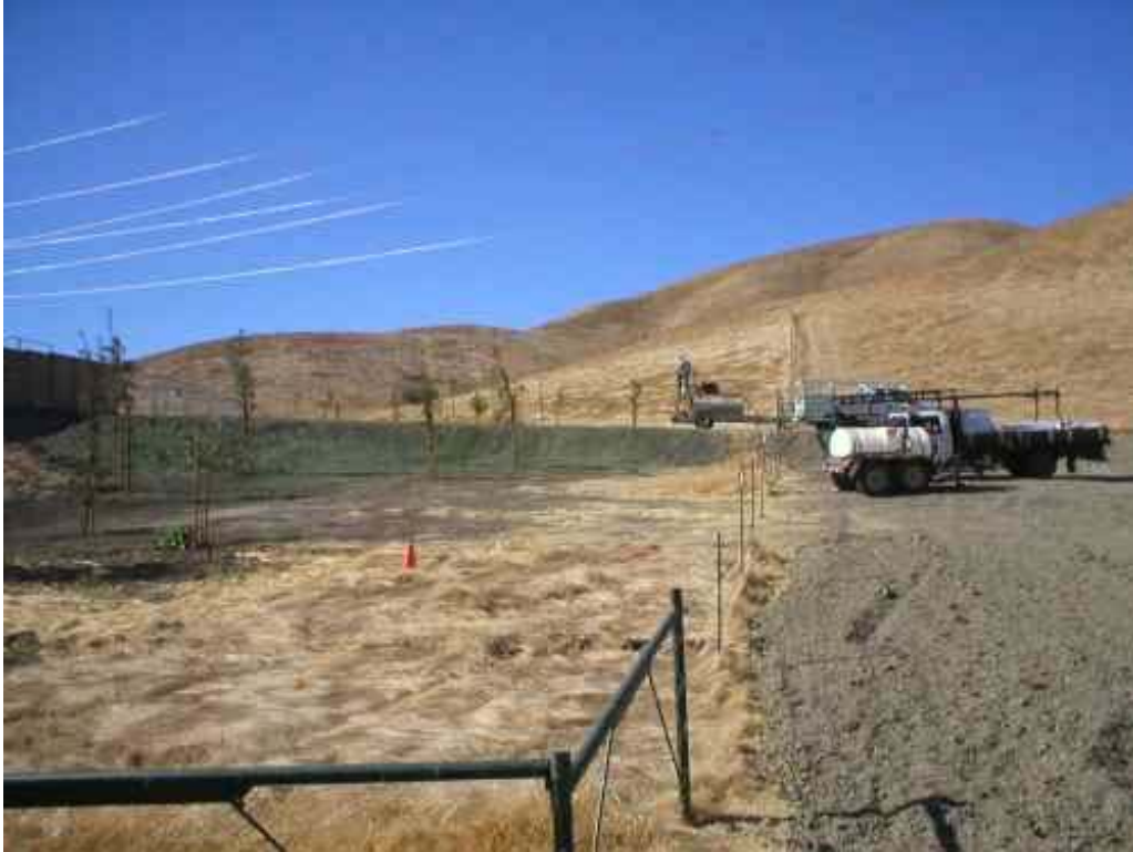
Figure 10 – NVC crews hydro-seeding the area around the North Dublin Substation pad, October 17, 2006.
