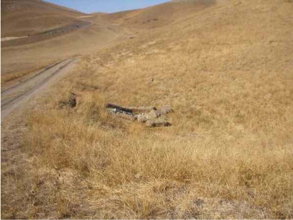
Figure 4 – Intact hay bales protecting a culvert area along Road 7, October 13, 2006.
