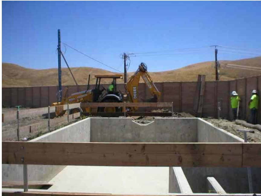
Figure 3 – Granite crews trenching for plumbing hookups to the SPCC pond at the North Dublin Substation, June 22, 2006.
