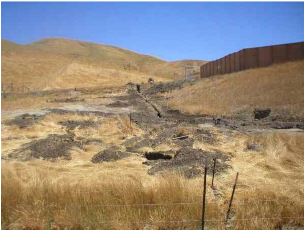
Figure 3 – Vitale and Sons installing irrigation line around the North Dublin Substation. July 11, 2006.
