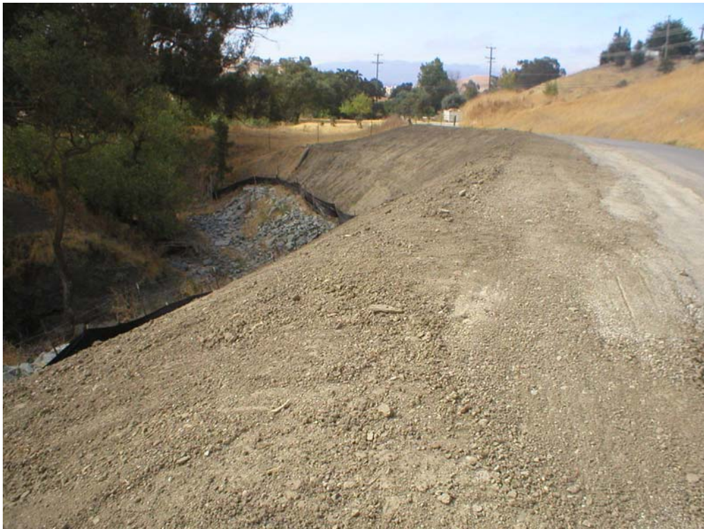
Figure 4 – NVC crews completed earthwork at the Tassajara Creek bank stabilization area, August 29, 2006.
