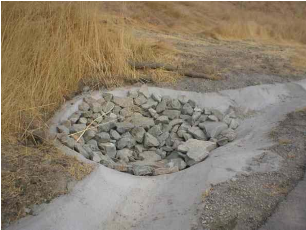
Figure 5 – Rocks have been replaced in the restored culverts along Moller Road, August 29, 2006.
