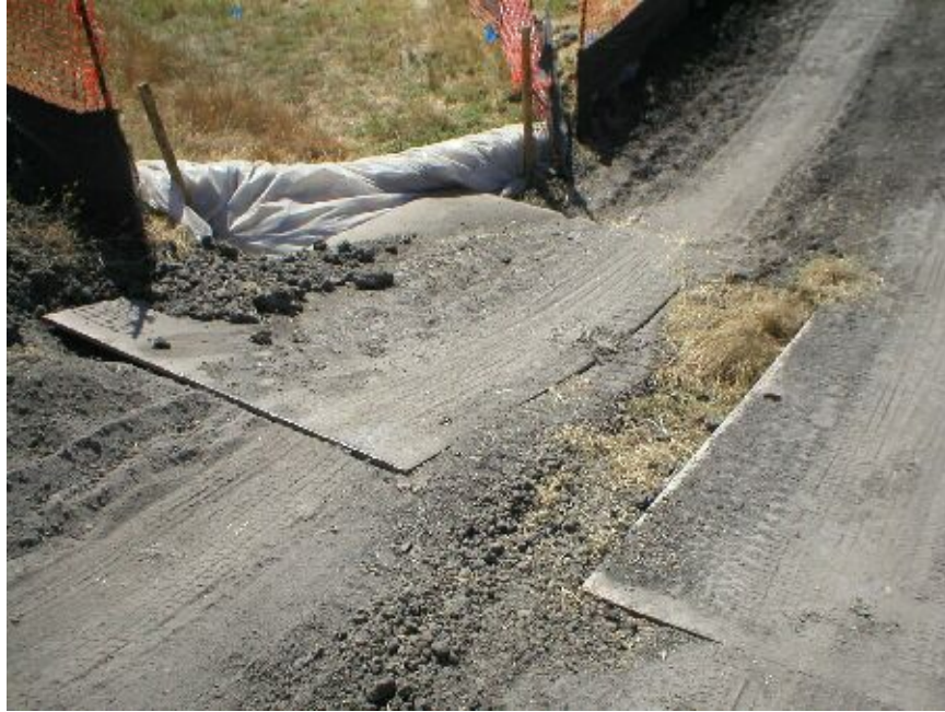
Figure 3 – Steel plate temporary bridge over Cayetano Creek, September 14, 2005. Note the spoils within the streambed.
