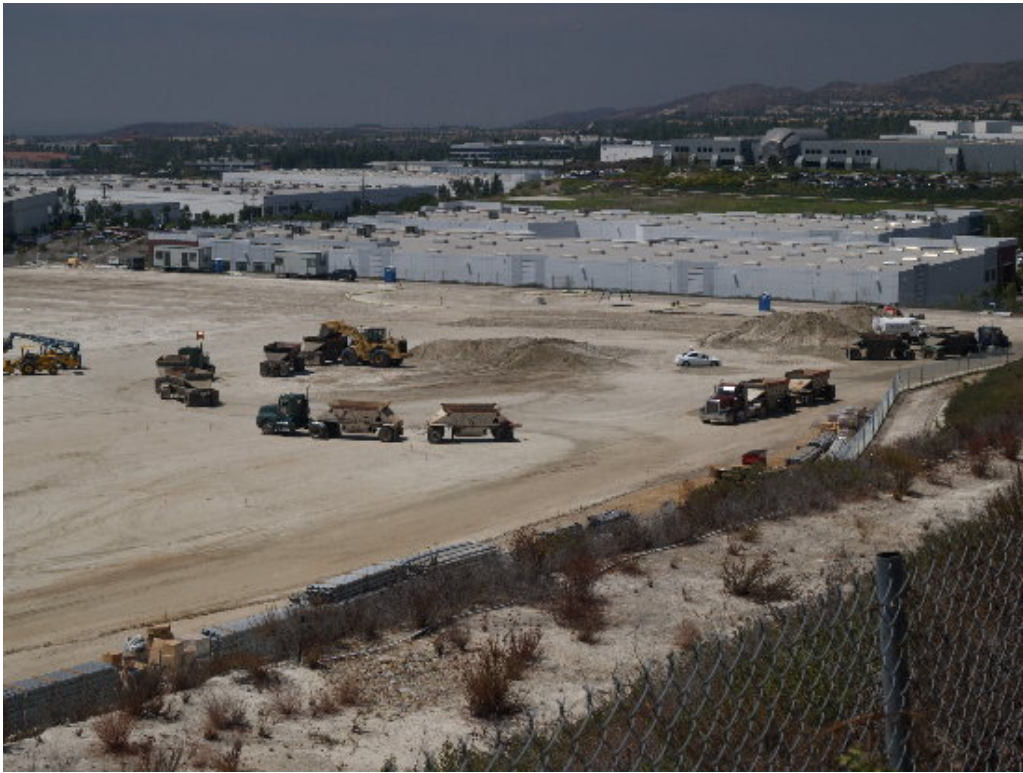
Figure 3 – Excess spoil from the right-of-way being loaded into trucks for removal from the substation site.
