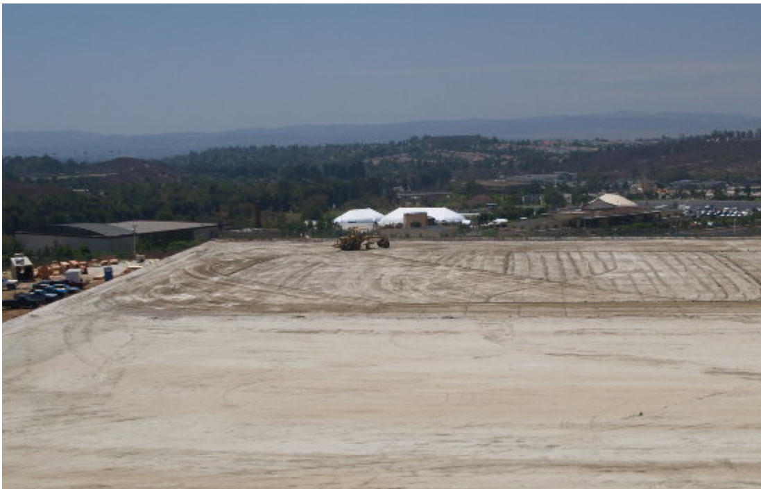
Figure 2 – An operator in a grader smoothed substation site after the completed grounding grid had been backfilled.
