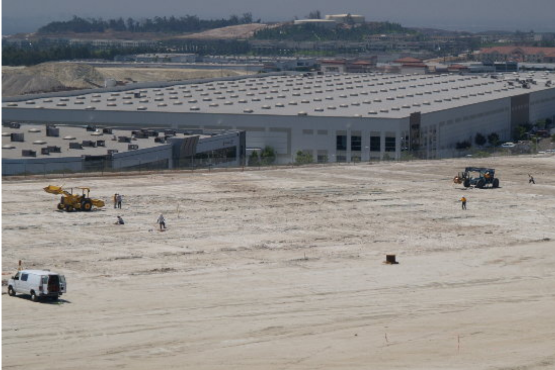
Figure 1 – Crew placing copper wire in the grounding grid on the substation site.
