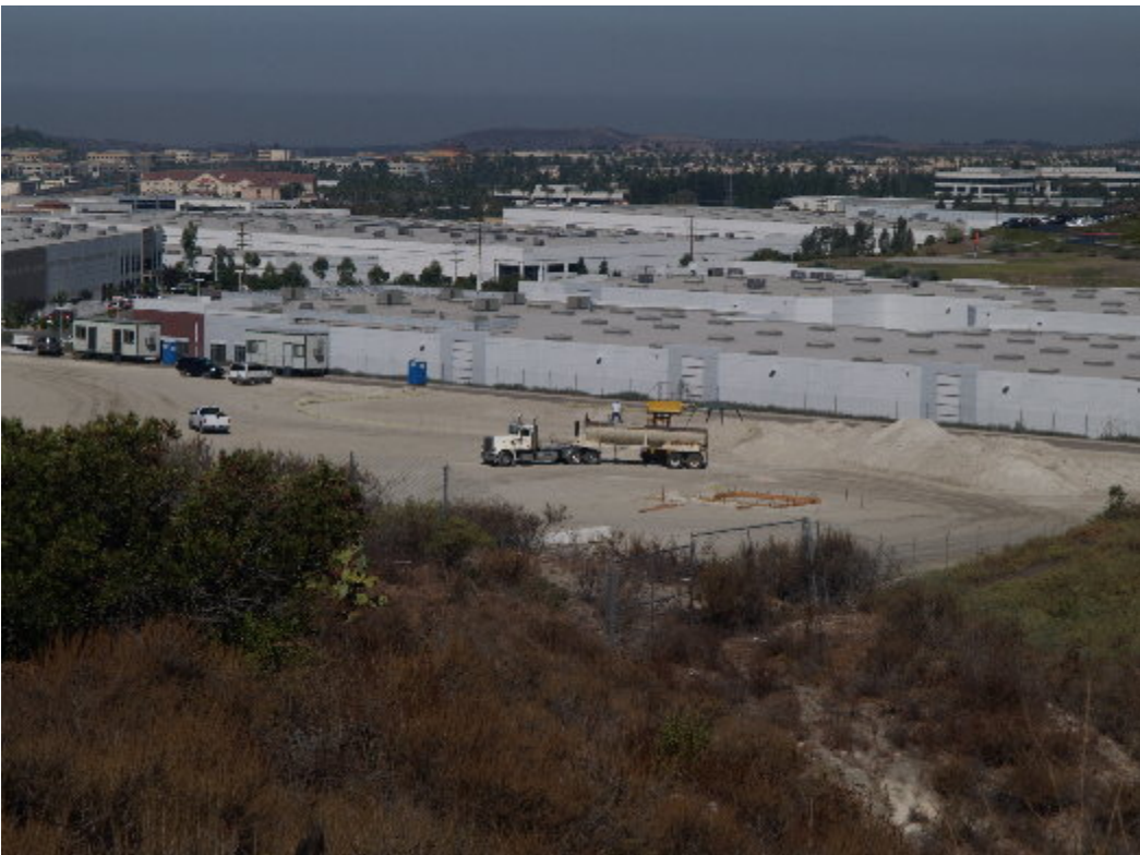
Figure 2 – An operator in a backhoe loaded excess spoils into trucks for removal from the station site.
