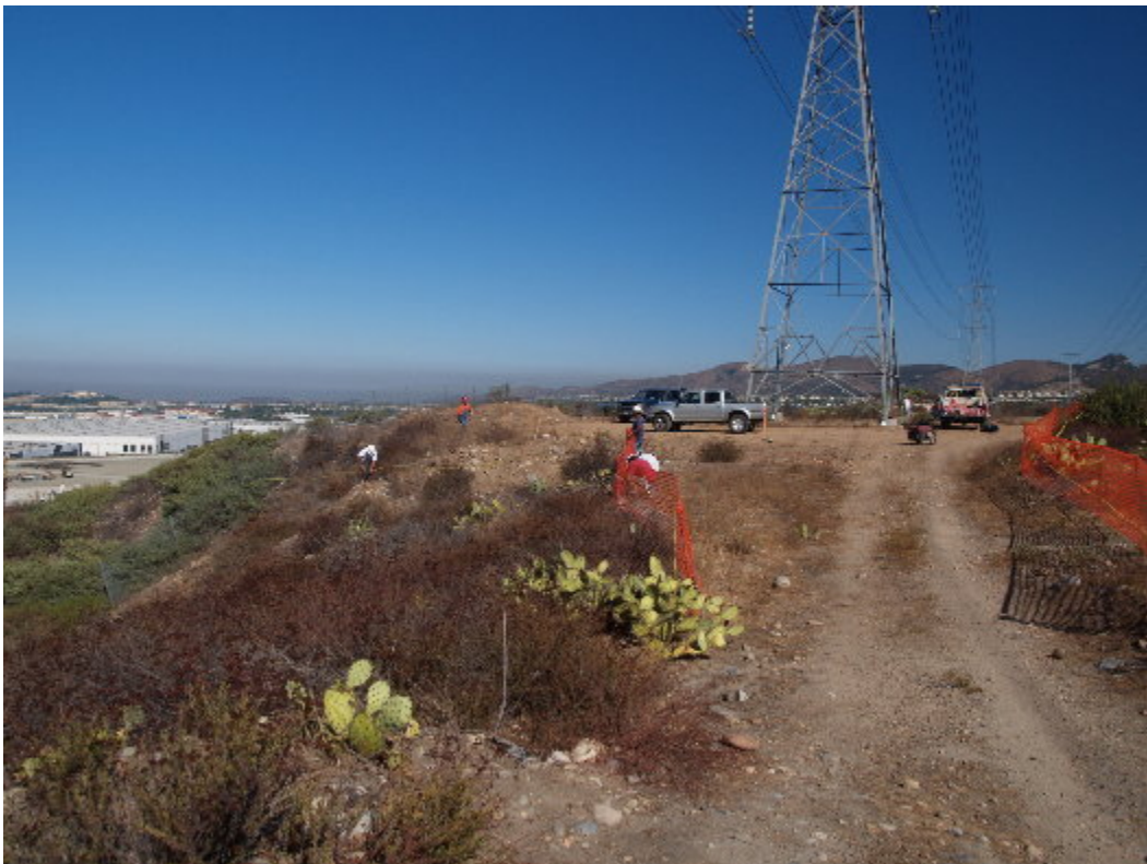
Figure 4 – Exclusion fencing was placed around the tower sites and work areas along the 230 kV transmission line corridor in preparation for the upcoming NTP.
