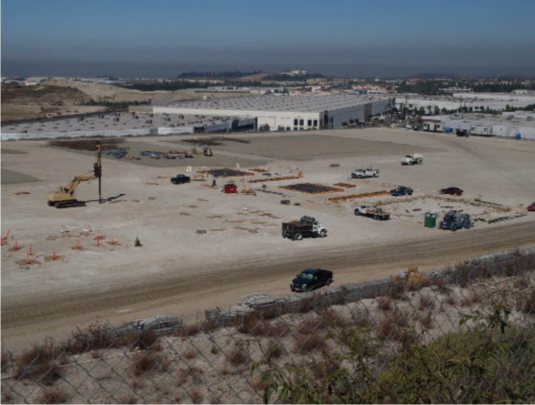
Figure 1 – Crews worked on the excavation and form work for the foundations on the substation site.
