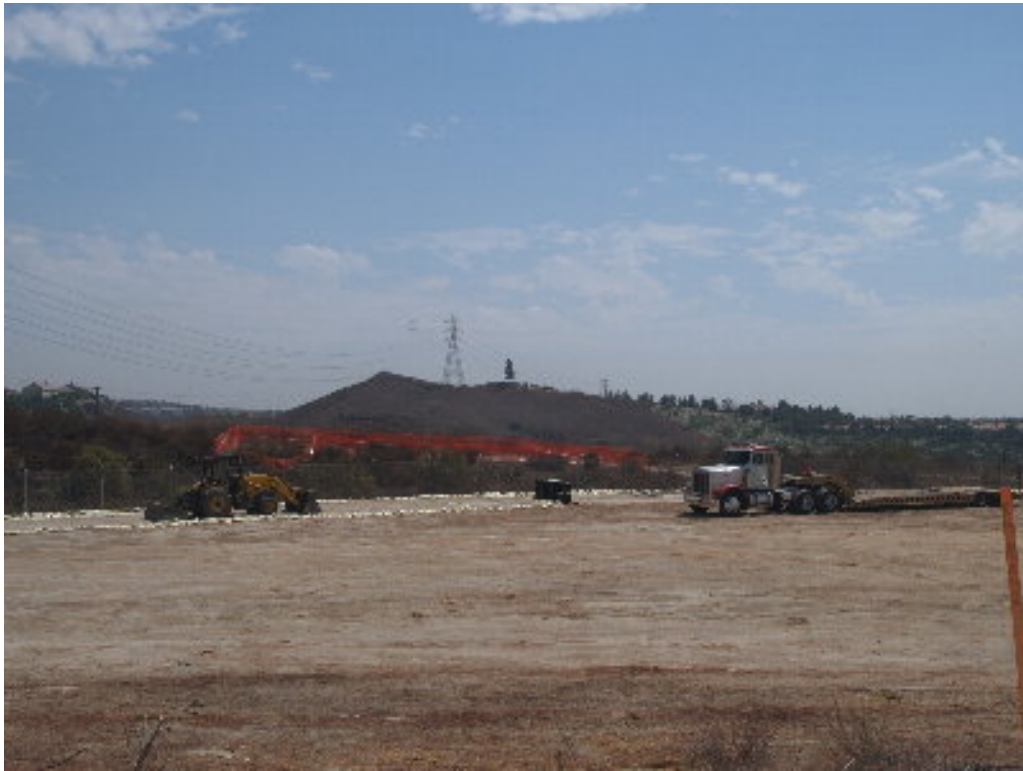
Figure 4 – Exclusion fencing has been completed at the tower sites and work areas along the 230 kV transmission line corridor in preparation for the upcoming NTP.
