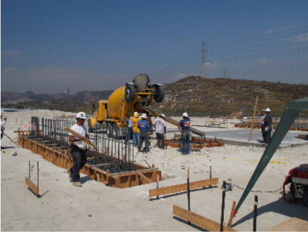
Figure 1 – Crews poured concrete into the completed form work for the foundations on the substation site.
