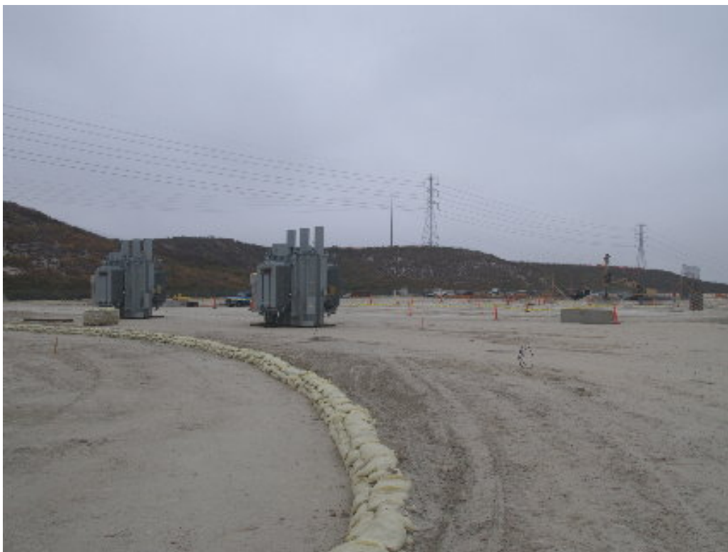
Figure 4 – The two B transformers (66 kV) have been delivered to the substation site.
