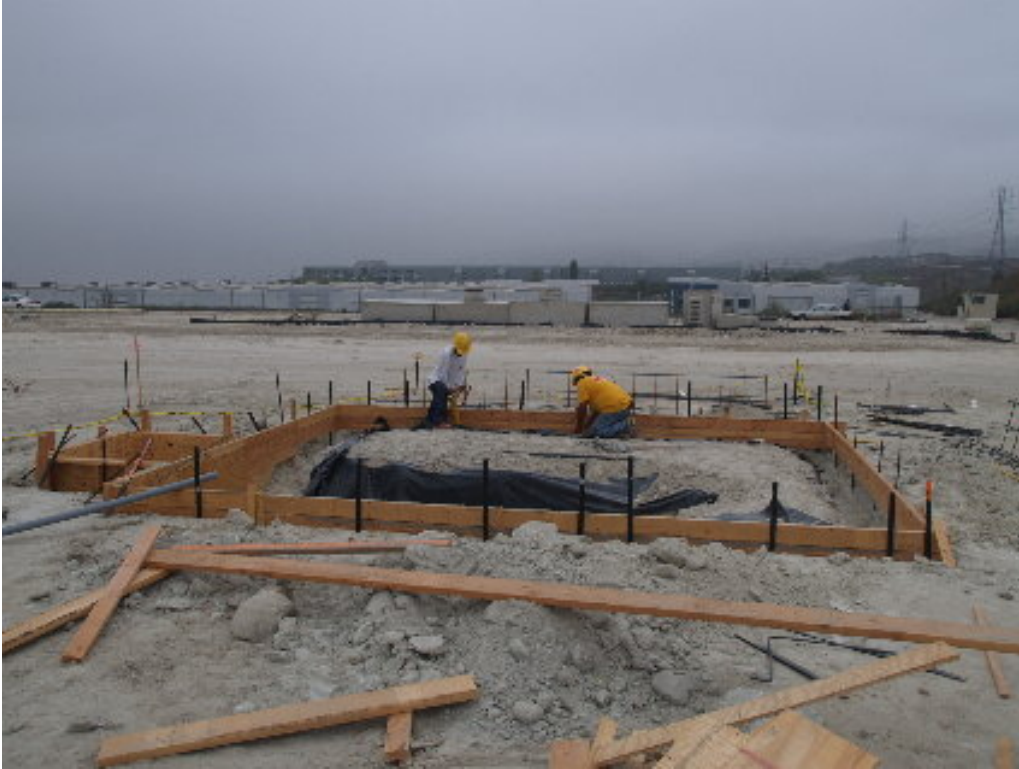
Figure 1 – Crews working on the form work for the foundations at the substation site.
