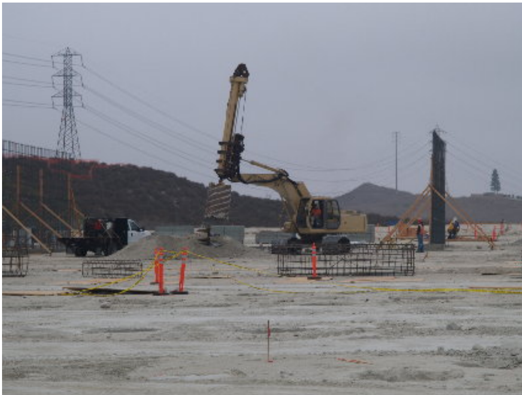
Figure 3 – Drilling continues between the vertical forms for the firewalls that will separate the two A transformers (230 kV).
