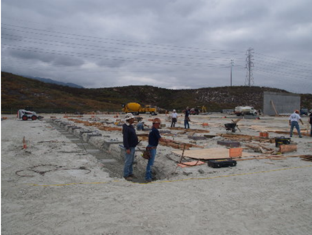
Figure 1 – Crews working on the grounding and foundation for the preformed concrete vaults.
