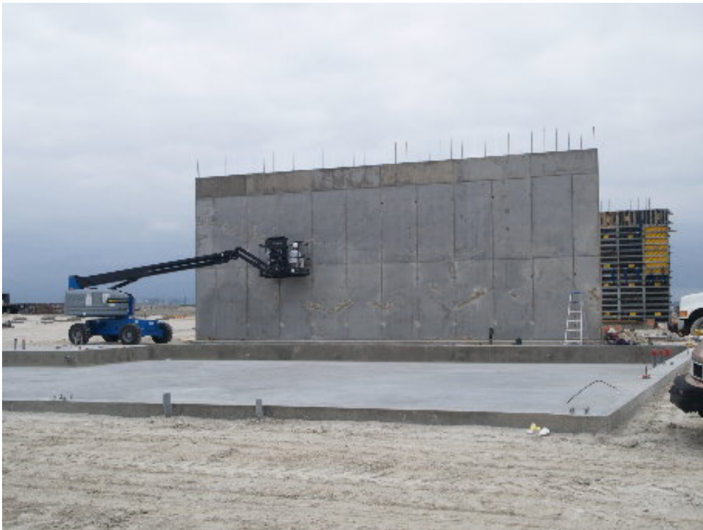
Figure 3 – Workers filled imperfections in the eastern firewall left from the reusable formwork. Cinderblocks will be added to the top where rebar protrudes.
