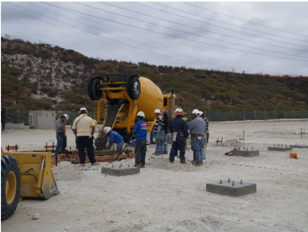
Figure 4 – The crew poured concrete into one of the 50 foundation forms that were ready.
