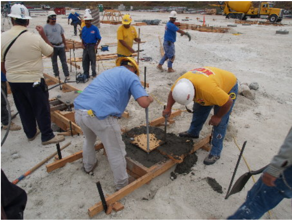
Figure 5 – Concrete workers placed small anchor bolts in the wet concrete prior to setting.
