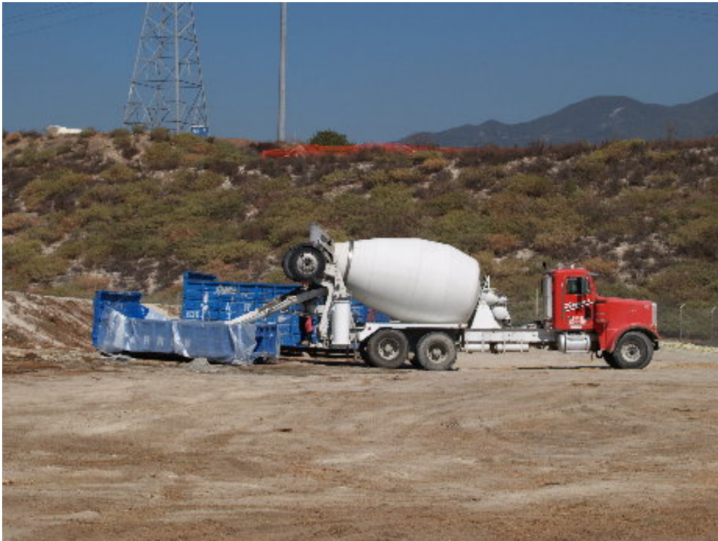
Figure 3 – Concrete trucks were properly washed at a lowboy dumpster set up in the southern laydown area.
