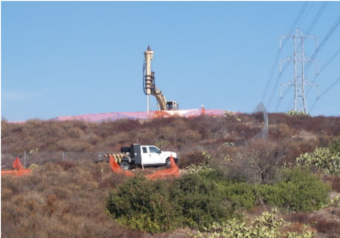
Figure 4 – Drilling of the tower foundations on the 220 kV section started during the subject week.
