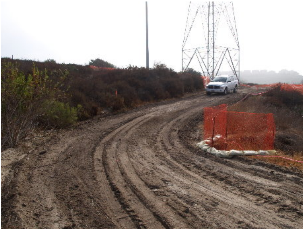
Figure 5 – A section of the access road for the 220 kV line has eroded and needs to be prepared for the safe passage of larger equipment.
