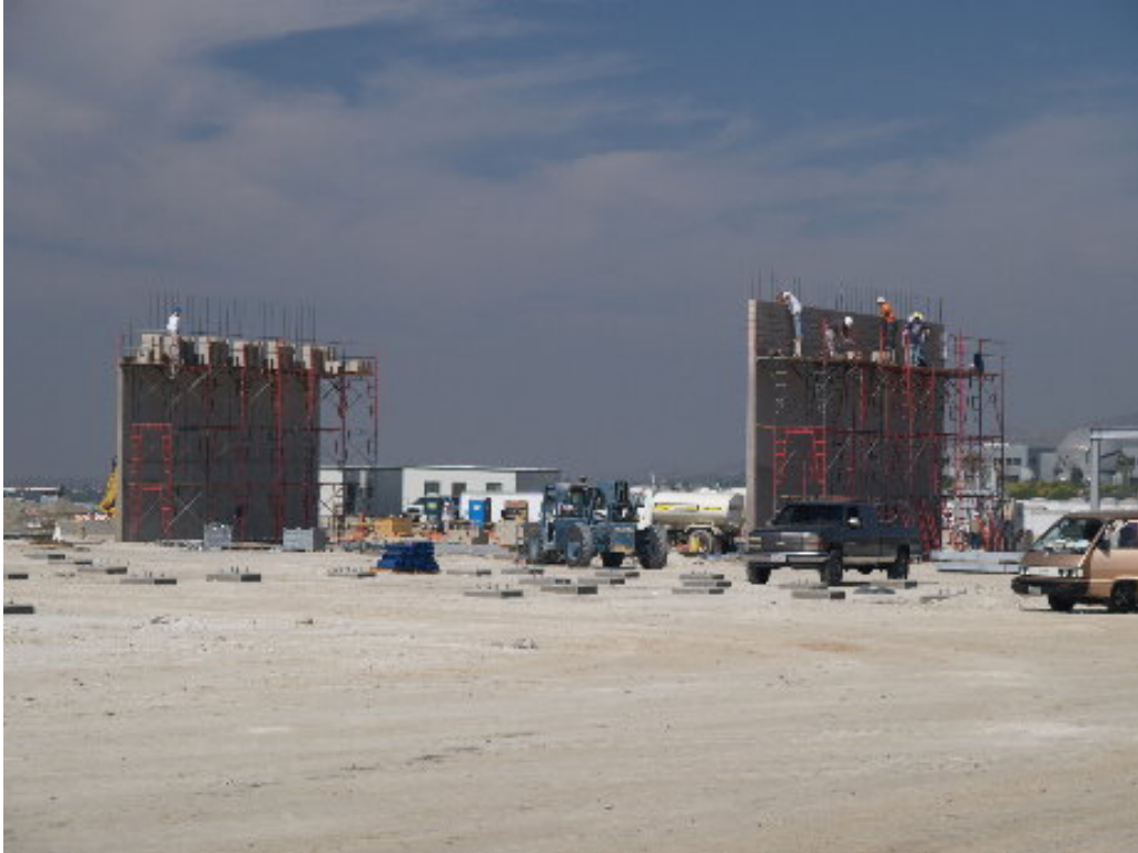
Figure 1 – The firewalls for the A transformers were poured and crews worked to top the walls with cinderblocks.
