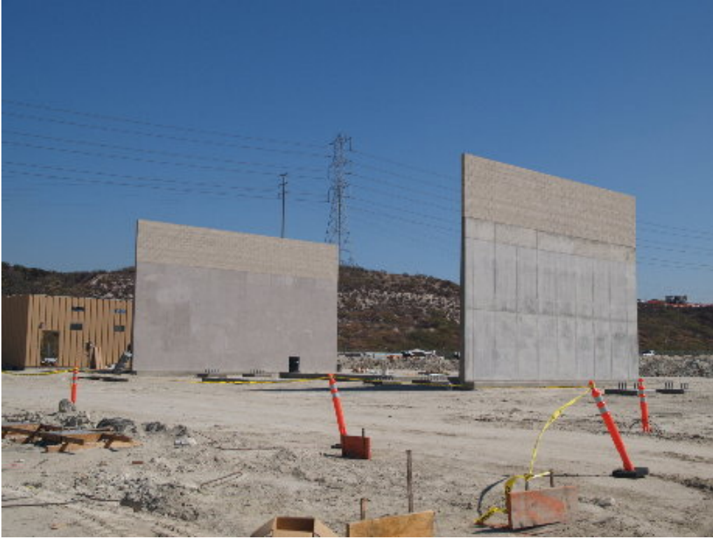
Figure 1 – The tops of the firewalls for the A transformers were completed with cinderblocks.
