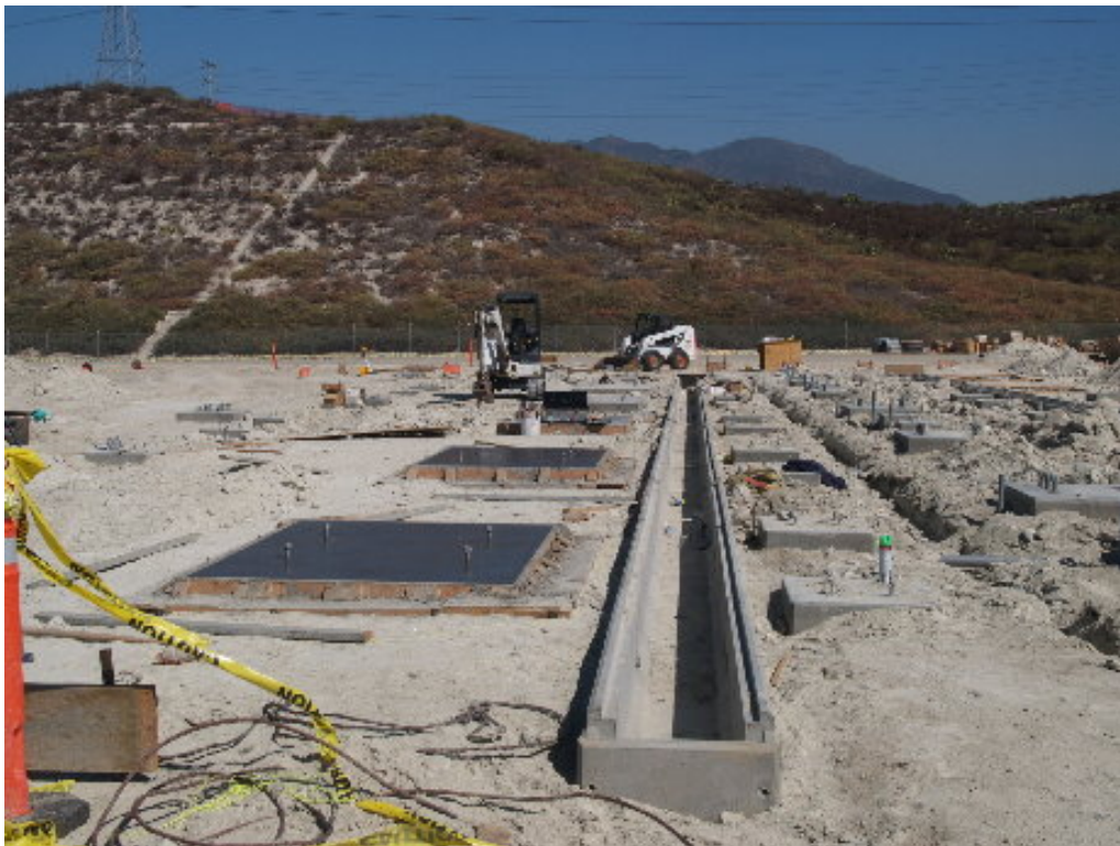
Figure 4 – A series of small pre-cast concrete trenches lead into the main trenches and then into MEER #1 or MEER #2. Pictured is the smaller trench for the 66 kV system.
