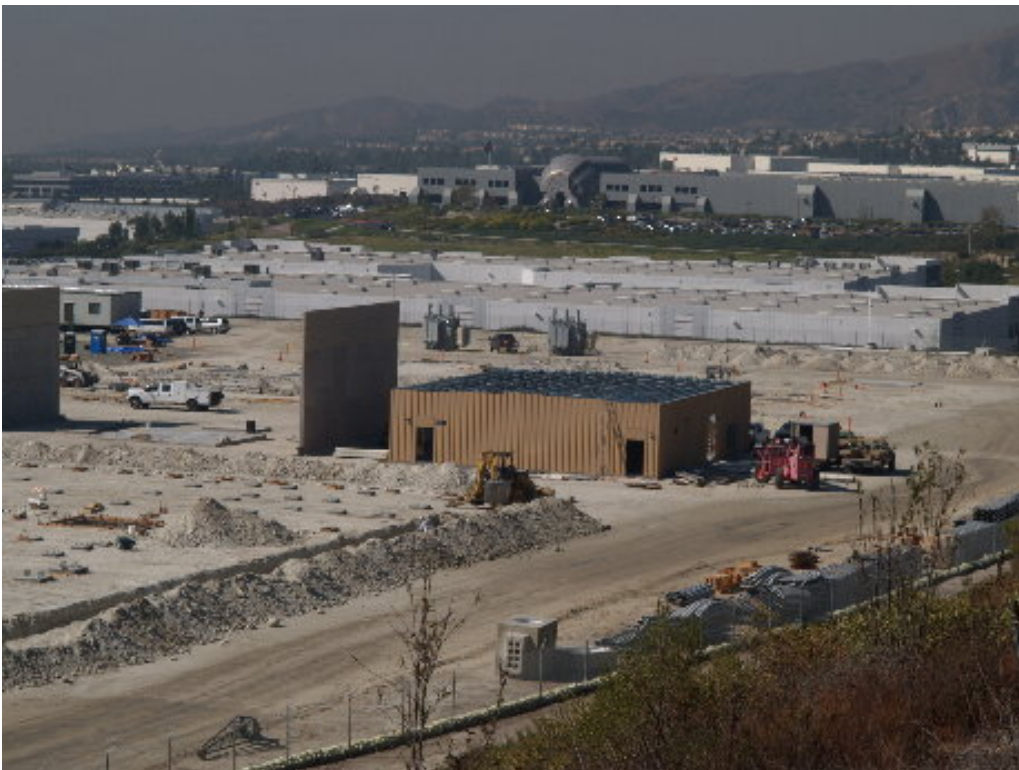
Figure 2 – A specialized crew installed the metal walls for MEER #1 during the later part of the week.
