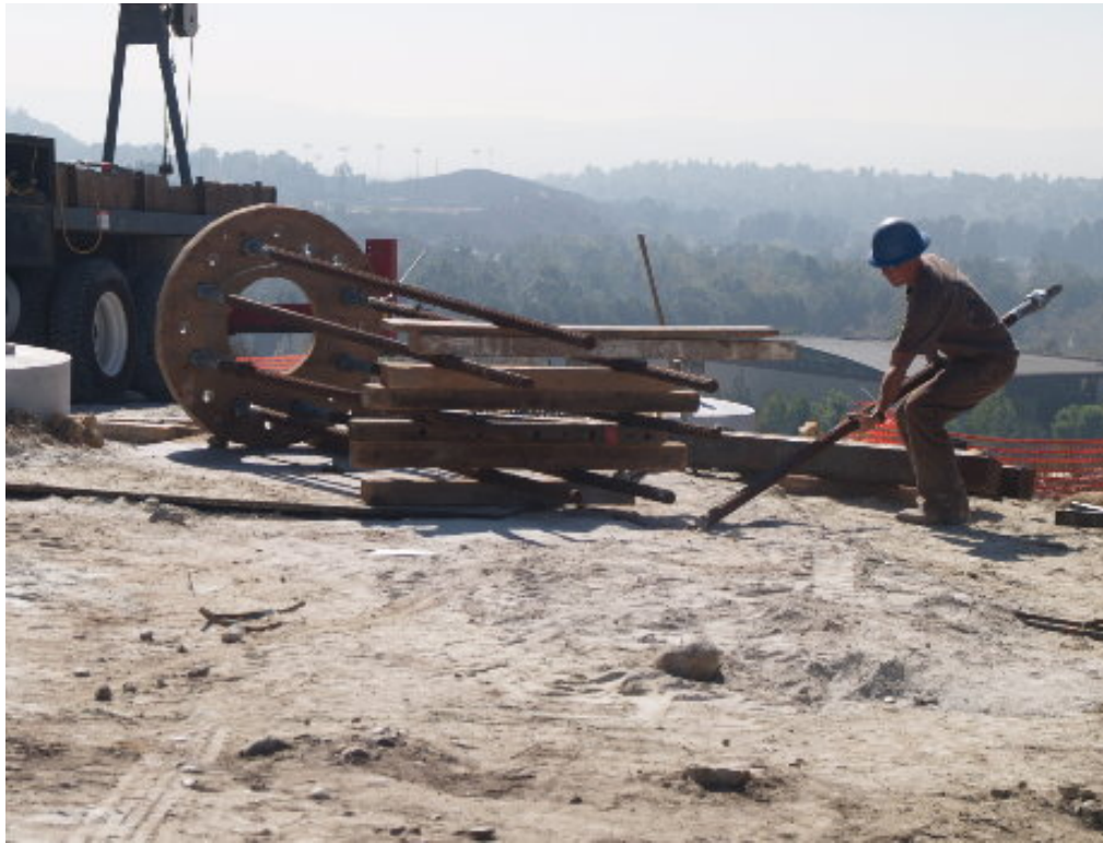
Figure 7 – A worker assembled the anchor bolts for the 220 kV foundations on the hill above the substation site.
