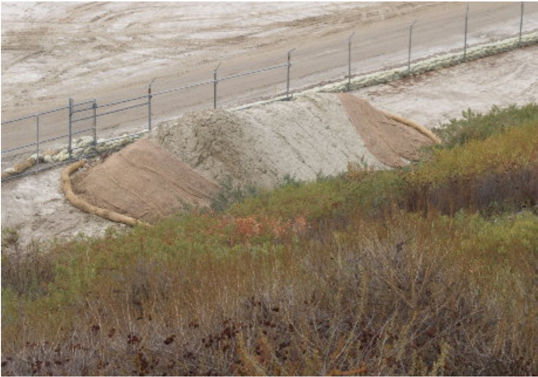
Figure 5 – The spoil pile for the pole foundation at the base of the hill adjacent to the south end of the substation site has been partially covered to minimize sedimentation.
