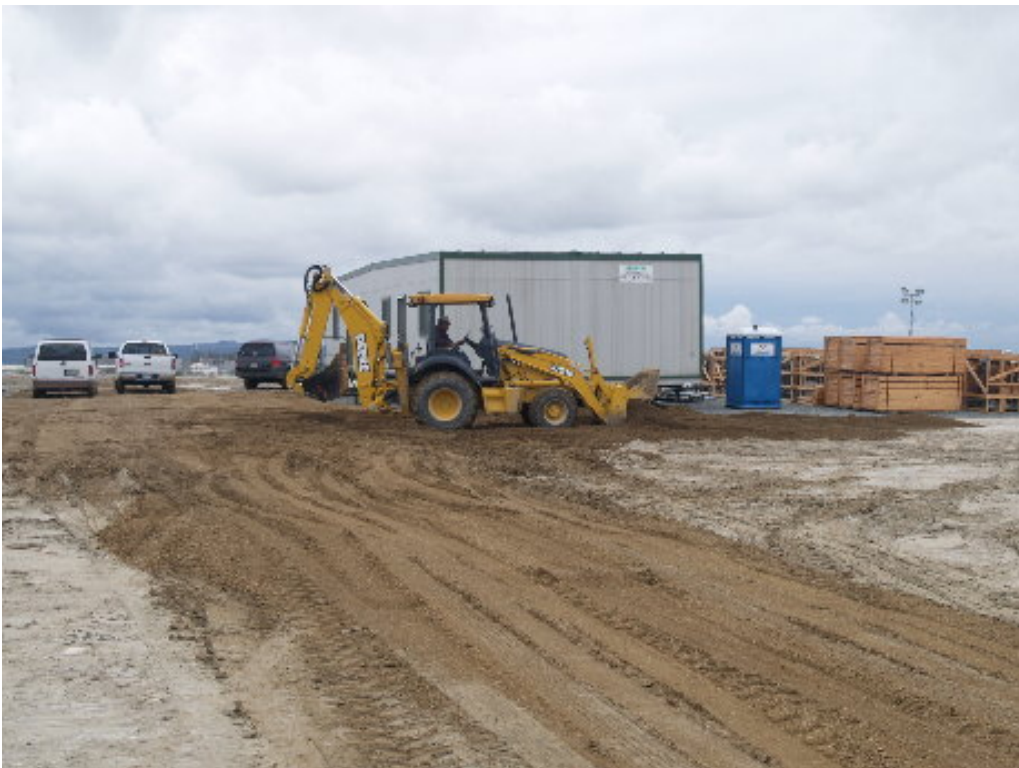
Figure 2 – An operator worked with a backhoe to place base rock on the access road and parking area for the construction trailers on the substation site.
