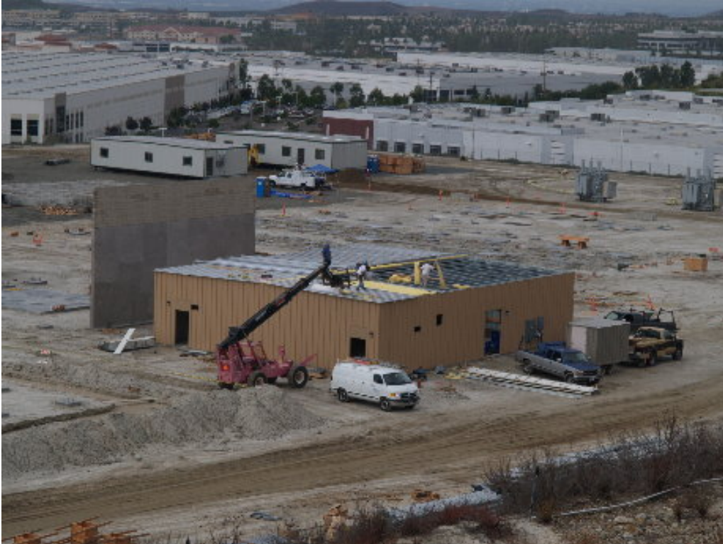
Figure 1 – A specialized crew installed insulation and worked on the roofing for MEER #1 during the week despite the rain.
