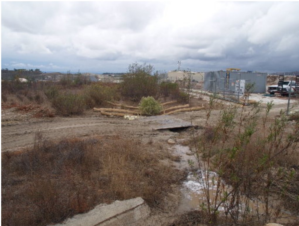
Figure 6 – Steel plates were installed on the access road for the 220 kV line to prevent vehicle traffic in the flowing water.
