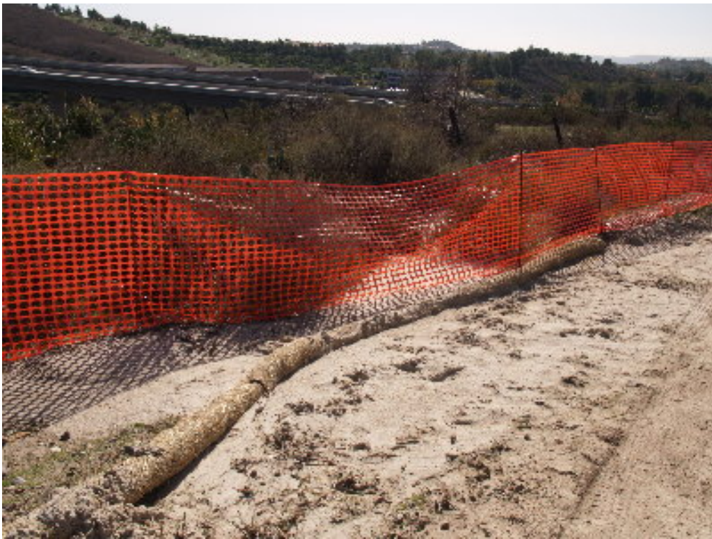
Figure 6 – Some of the straw wattle sediment barriers on the 220 kV transmission line have been overwhelmed by recent sediment and need maintenance and possible upgrading.
