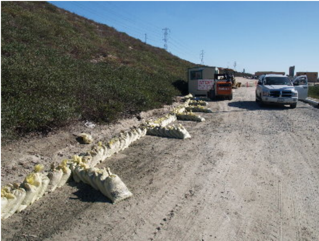
Figure 3 – The rows of sandbags placed near the guard shack were replaced and sediment removed.
