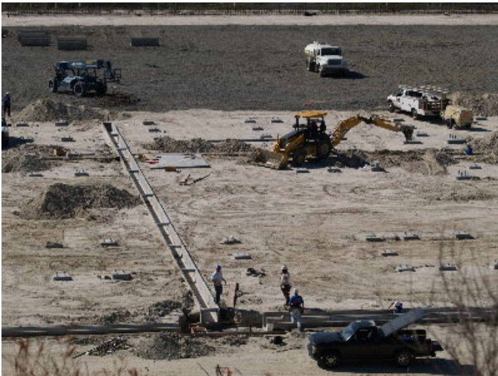
Figure 2 – Crews worked on excavation and preparation of the pre-cast concrete electrical trenches on the substation site.
