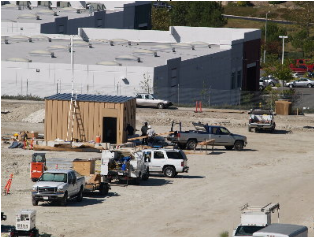
Figure 1 – The smaller 66 kV MEER #2 has been erected on the foundation and the specialized crew worked on the exterior sheet metal.
