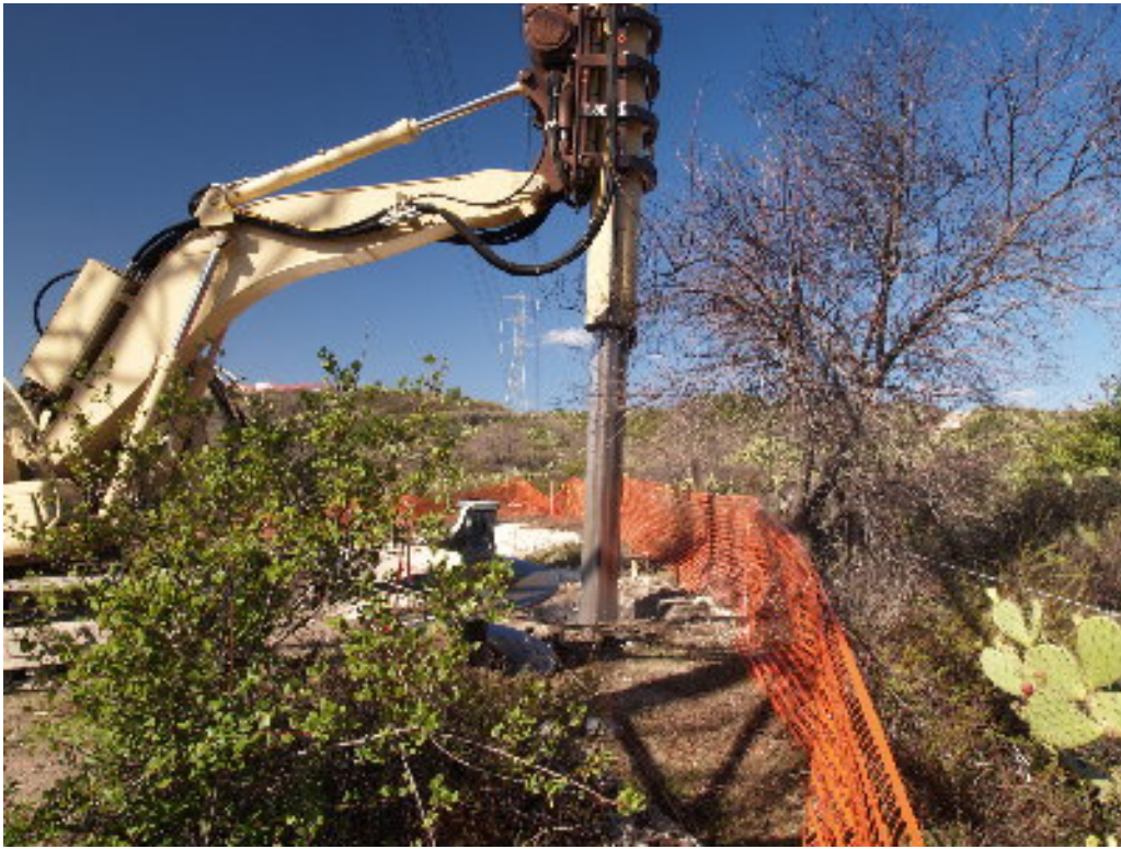
Figure 5 – The drilling crew worked on several foundations at the base of the hill southeast of the substation site.
