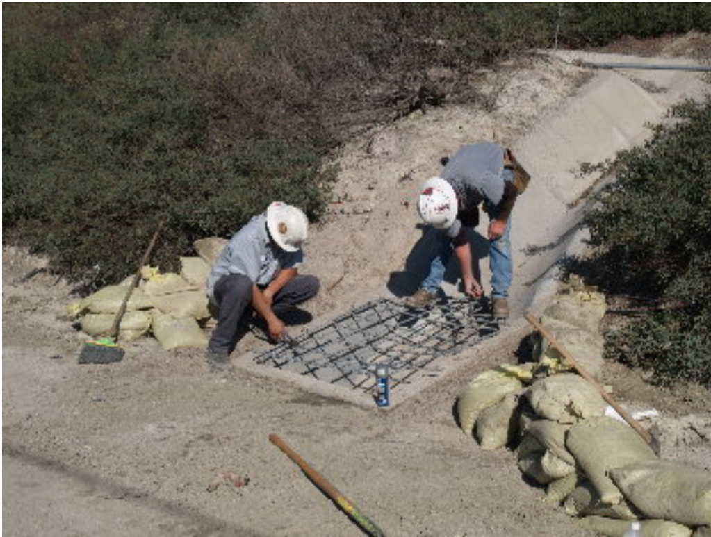
Figure 4 – The grate north of the guard shack on the access road was repaired so that filter fabric could be installed properly.
