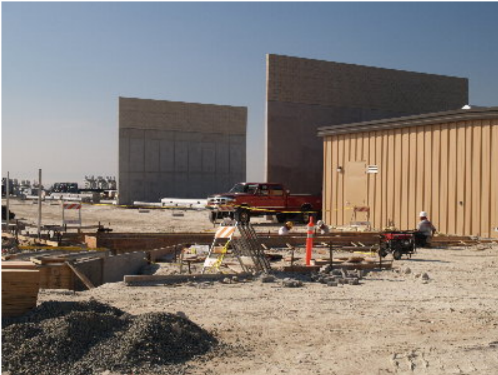
Figure 1 – Crews worked on the forms for the concrete section linking the pre-cast concrete trenches to the MEER #1.
