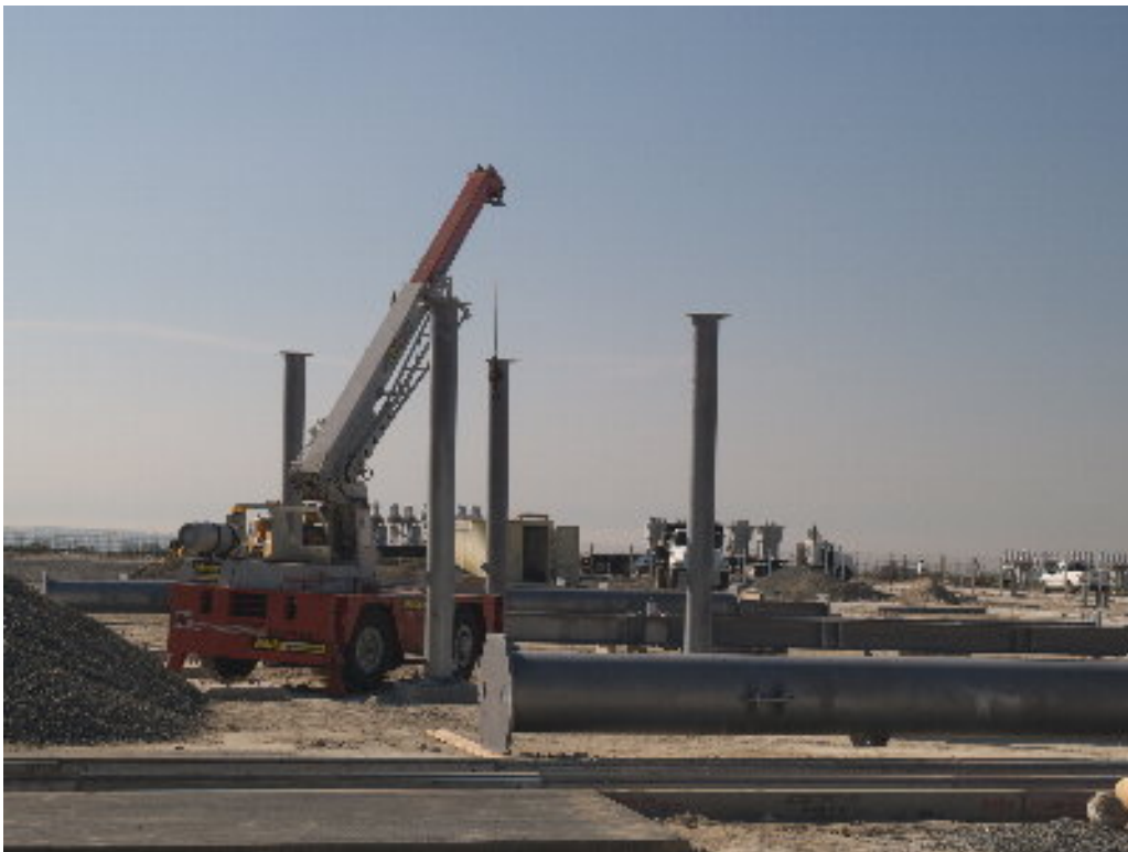
Figure 4 – A small crane was used to raise the supports on the southern end of the substation site.
