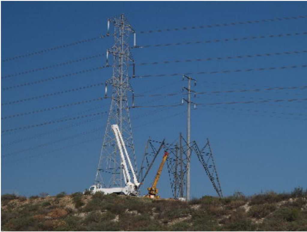
Figure 7 – The lower section of the middle lattice structure on the 220 kV transmission corridor has been completed.
