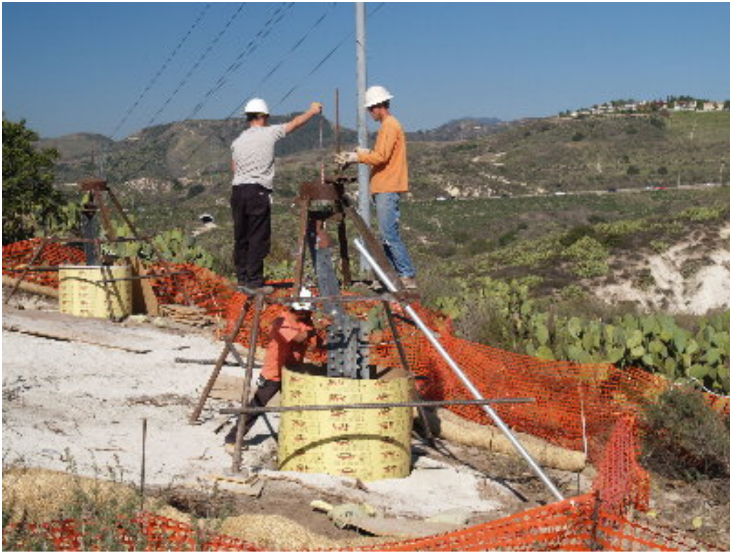
Figure 5 – A crew set the stub angles for the northern 220 kV lattice tower foundations.
