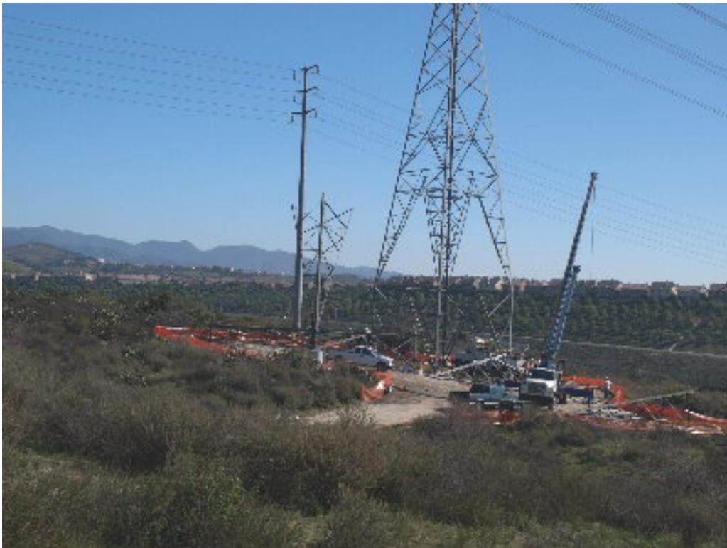
Figure 6 – Crews started erecting the lattice tower at the base of the hill southeast of the substation site.
