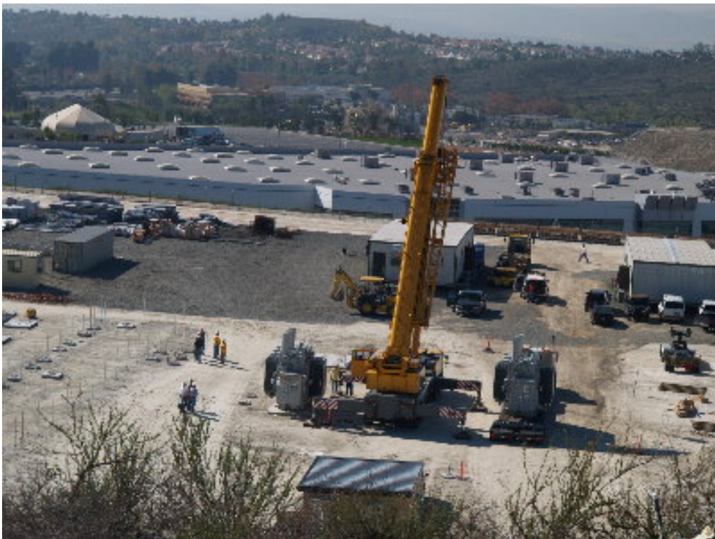
Figure 2 – A 300-ton crane was used to place the B transformers onto foundations.
