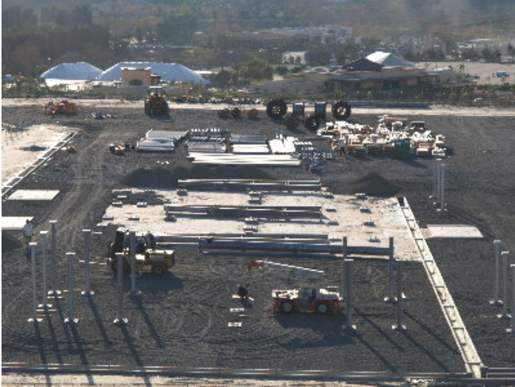
Figure 1 – A small crew worked on the supports on the southern end of the substation site.
