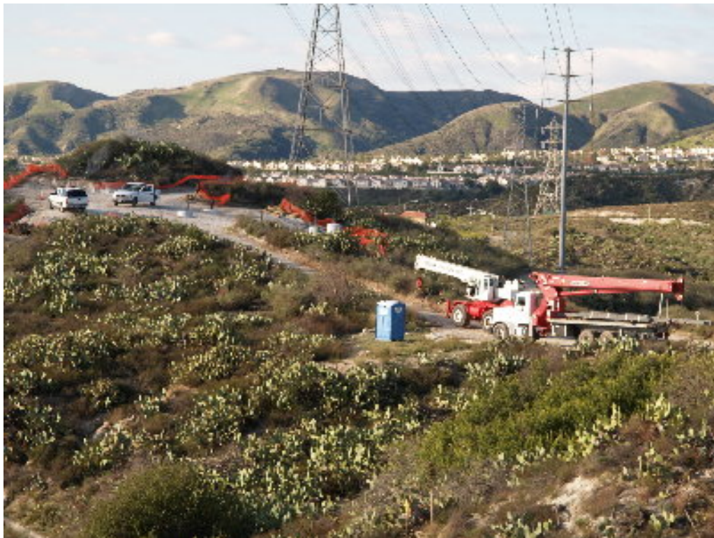
Figure 4 – The foundations were completed on the northern 220 kV tower and a small crane brought on-site to unload the steel for the lower tower section.
