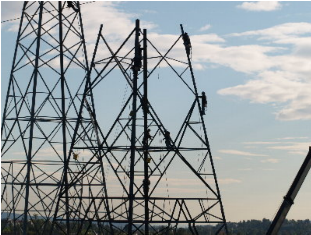
Figure 5 – Specialized crews continued erecting the lattice tower at the base of the hill southeast of the substation site.
