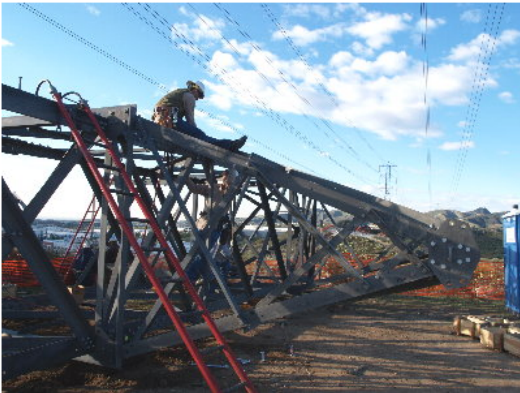
Figure 6 – Crews worked on the ground to assemble the upper section of the middle lattice structure on the 220 kV transmission corridor.
