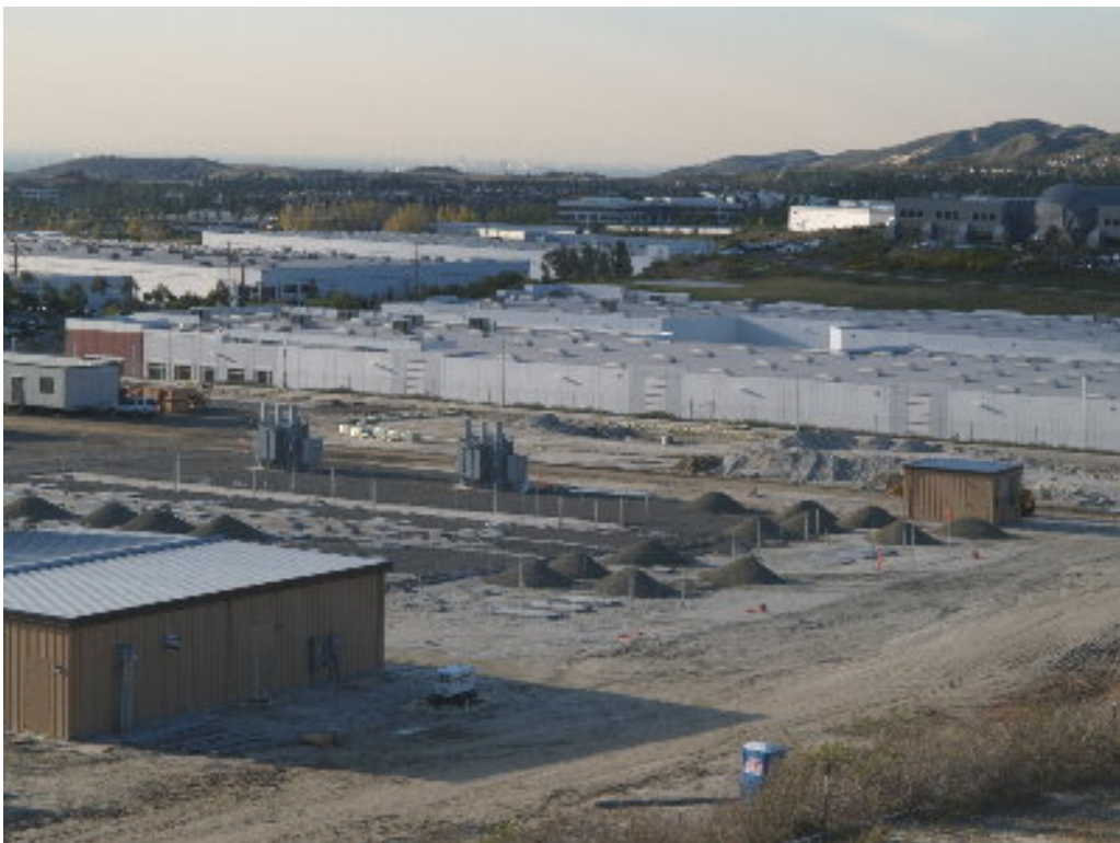
Figure 2 – Gravel piles were stockpiled on the northern end of the substation site while trenching is completed.
